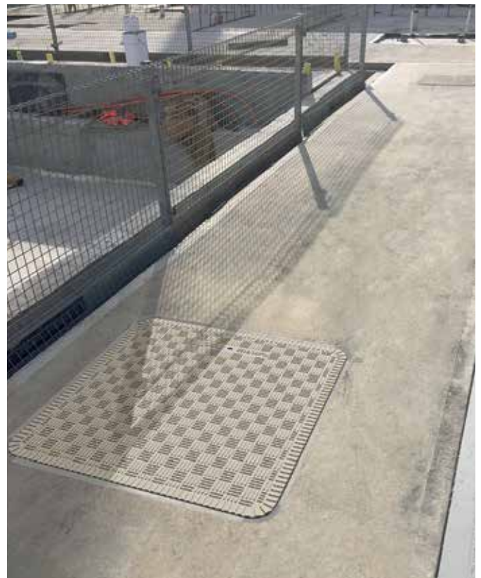
Installed cover over balance tanks
