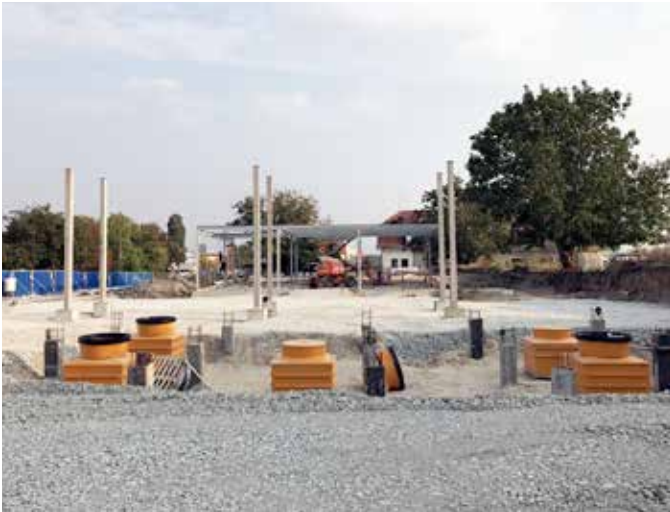
Fibrelite S7-390 GRP tank sumps require minimal maintenance and provide maximum protection (Photo taken prior to KPS pipe installation)
