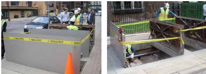
Previously installed aluminum covers - known for conducting heat to the surface
