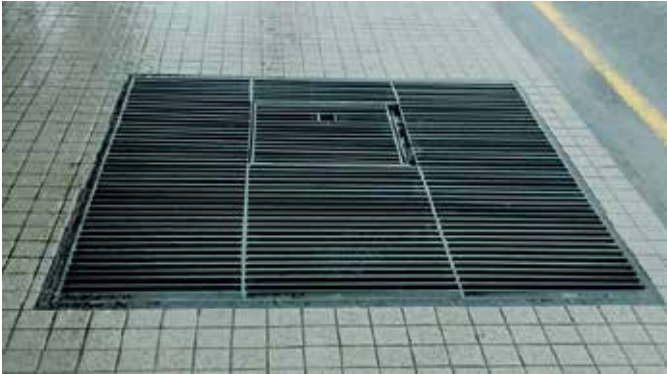
Metal covers causing a trip hazard for pedestrians
