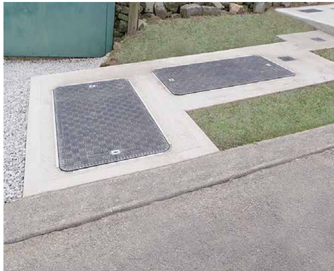
The 25 tonne load tested lightweight covers
