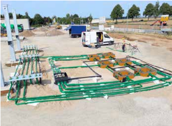
BP-Aral specified KPS' plastic double wall piping at a new build site in Hildesheim, Germany
