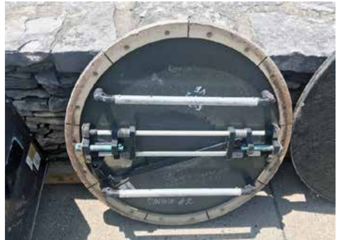
The adverse conditions of the steam vaults had caused the locking mechanisms to fail
