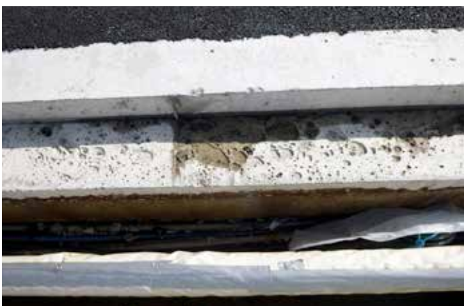
Custom sized covers were required to fit the unusual shape of the trench
