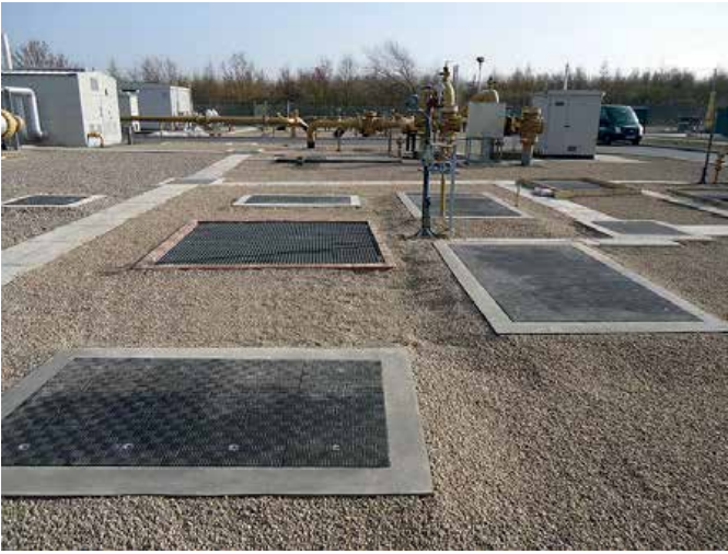
Corroded and damaged cast iron and concrete covers were replaced with Fibrelite's lightweight trench panels
