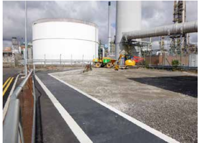
Fibrelite covers have resistance to extremely high temperatures and so can withstand the emissions from the steam pipes below them
