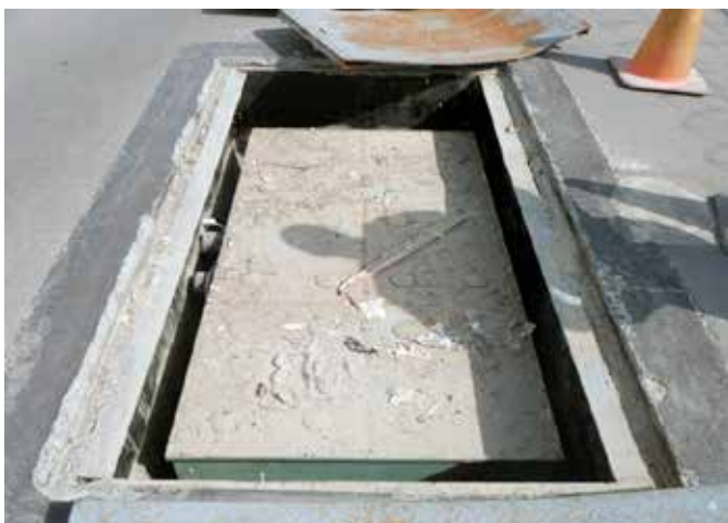
Previously installed chequered metal plate covers had deformed due to HGV traffic
