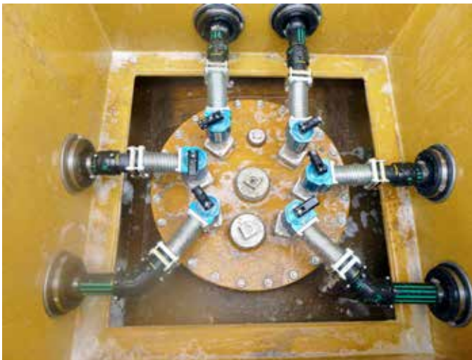
The Fibrelite site team conducted a vacuum test on site after the install
