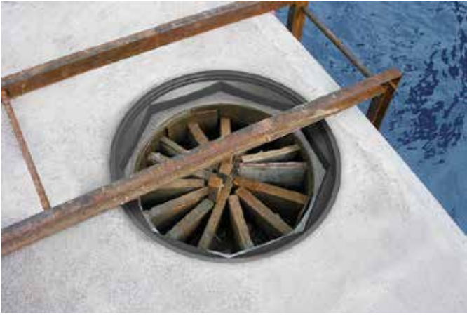
Composite frame over fresh water valve pit in concrete
