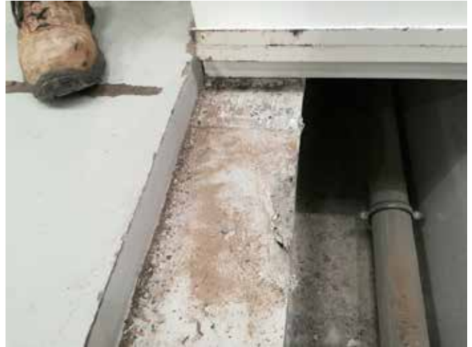
Uneven trench recess depth
