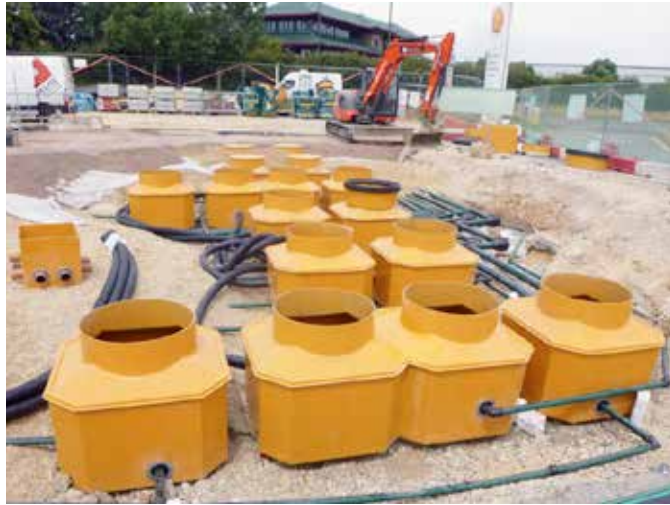
Bespoke Fibrelite chambers installed at Shell Eastfield
