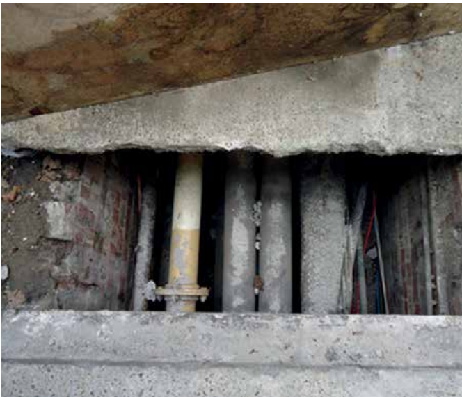
Removed crumbling concrete cover showing heating pipes underneath
