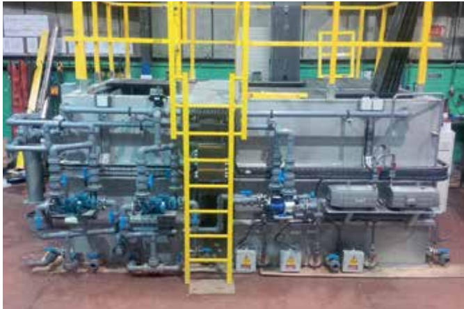
The specialist waste water treatment system at this plant
