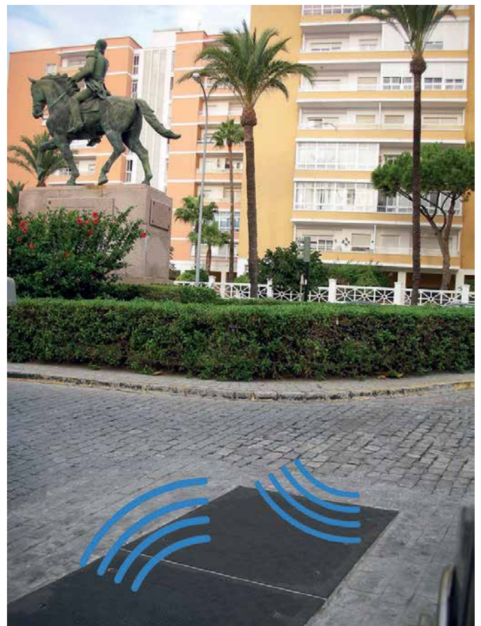
Fibrelite FM45 covers installed allowing RF signals to pass freely through (Image credit: Aguas de Cádiz)
