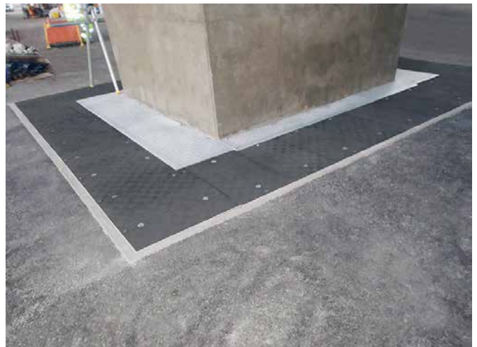
Replacement bearings located in the underground pits, covered by continuous set of access covers, allowing for the minor movement of the pier
