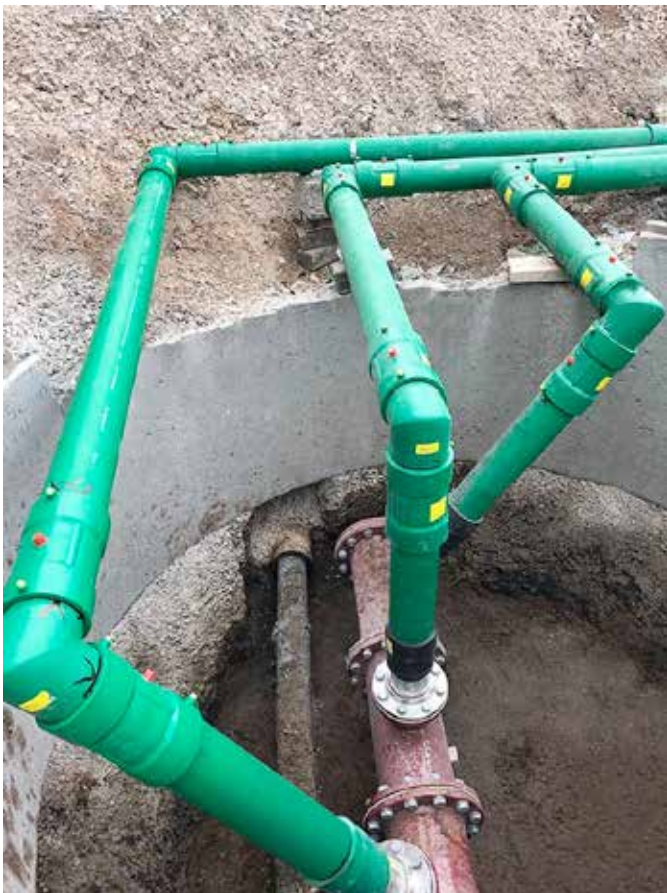
Compact moulded elbows make the join from new KPS piping to the previously installed fuel piping
