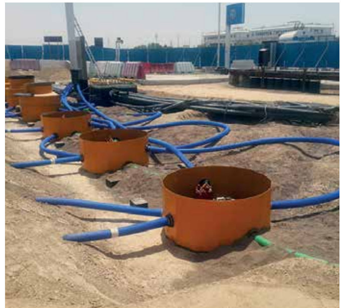
Fibrelite tank sump system with pipework attached using Fibrelite pipe entry seal kits, forming a watertight seal
