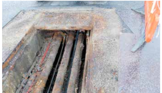
Previously installed failing concrete and metal covers
