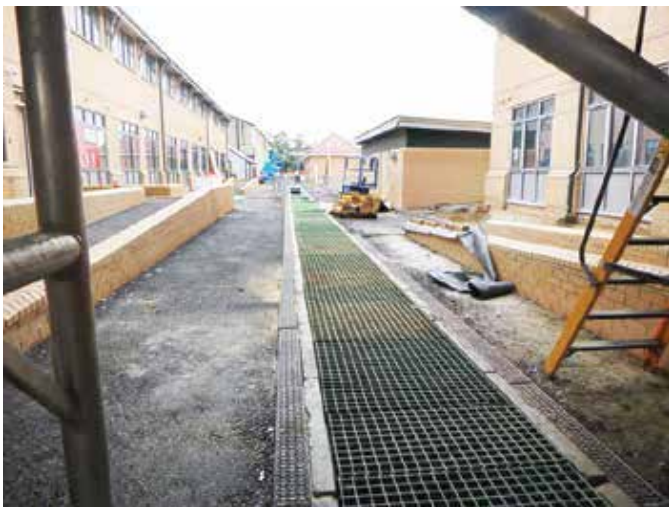
Previously installed GRP grating was unsuitable for sustained loading
