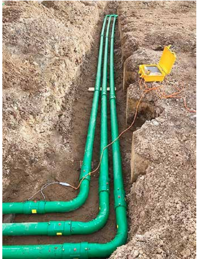
KPS double wall diesel piping
