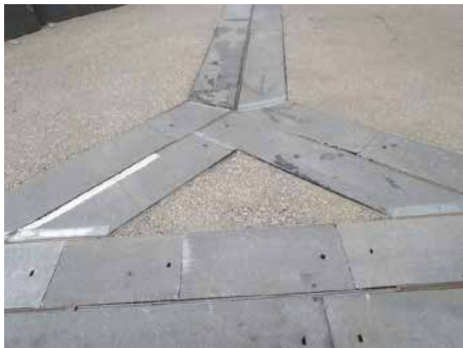
Existing covers had no tread pattern, potentially causing their surface to become slippery when wet
