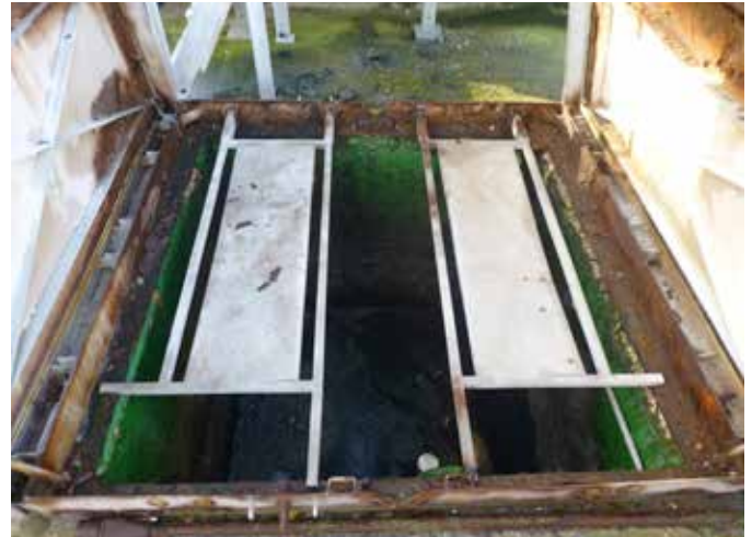
The old heavy mechanical steel covers were replaced with the Fibrelite lightweight alternative
