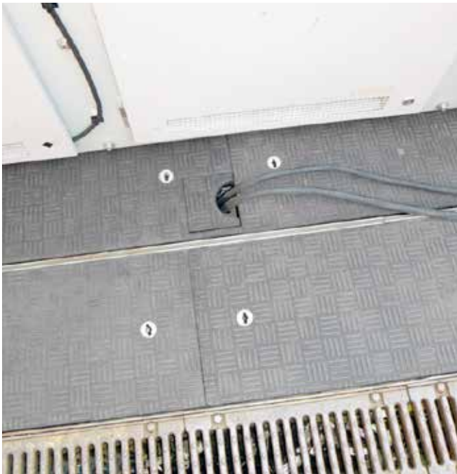
Fibrelite provided a retrofit solution which could be installed directly into the existing framework and provide the necessary interchangeable cable outlet arrangement without having to modify the Fibrelite covers
