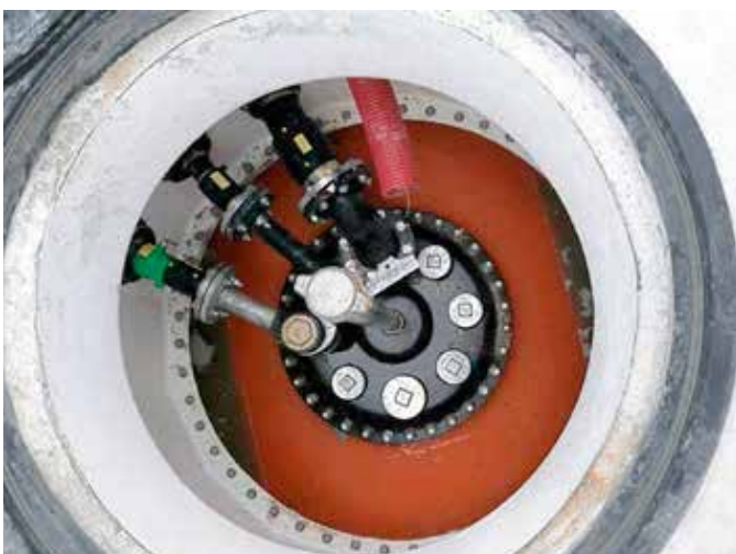
Control and monitoring of the interstitial space between the inner and outer pipes, provided an extra layer of security
