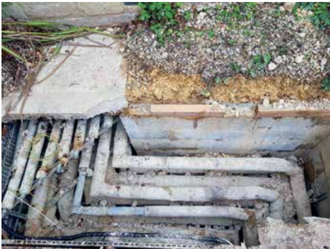
Previously installed concrete covers had fractured and chipped
