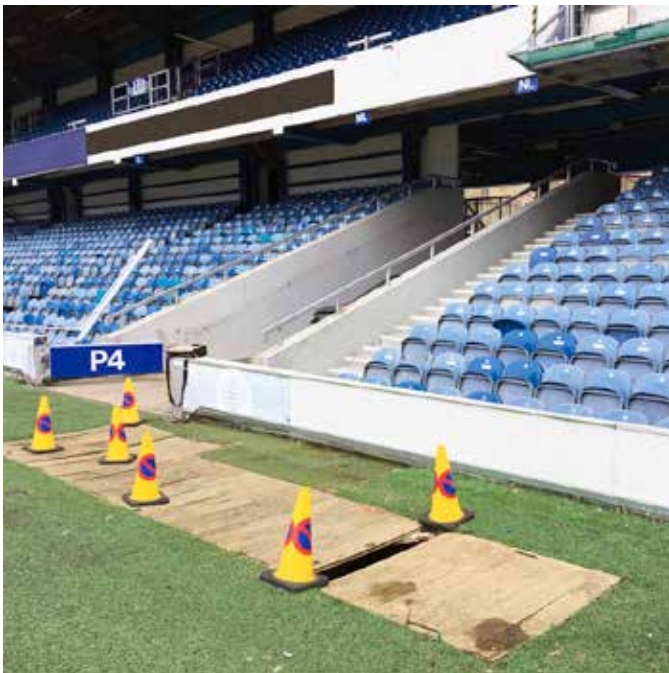
The previously installed makeshift plastic decking had been deemed unsafe for pedestrian use
