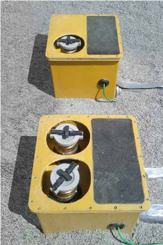
Secondarily contained Fibrelite remote fill sumps with anti-slip step down platforms
