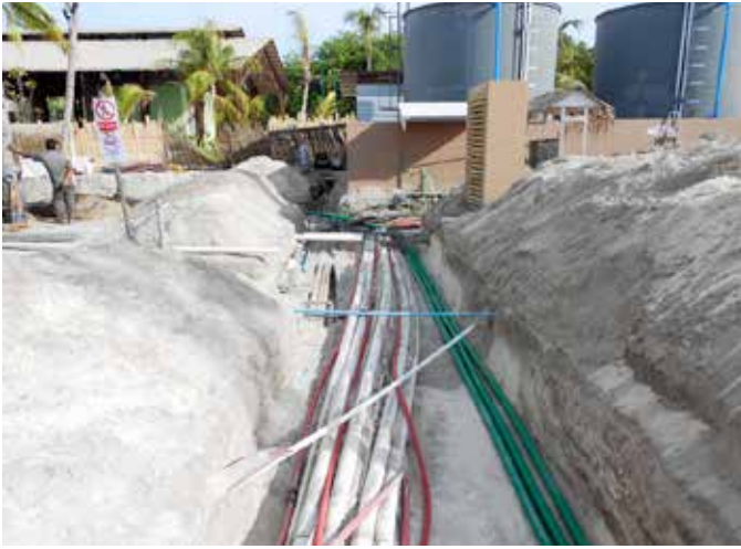
Fuelling lines running from jetty to storage point
