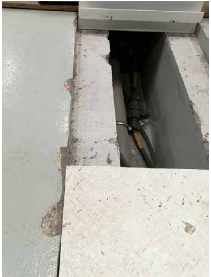
An uneven recess had destabilised previously installed covers
