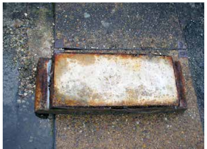
Corroded previously installed cover hinge
