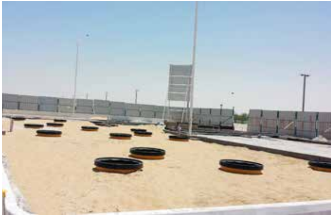
Fibrelite tank and dispenser sumps specified by Qatari oil company
