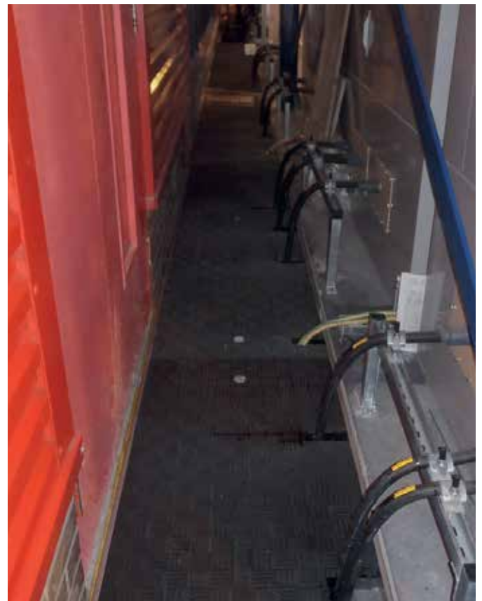
Trench panels cut and re-sealed on site allowing cables to run through
