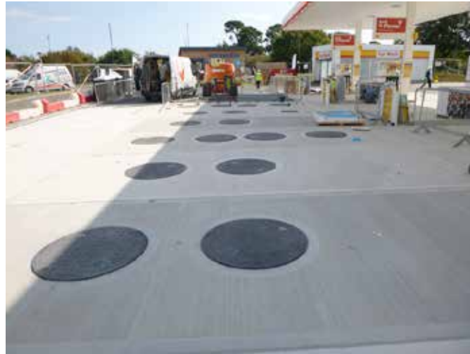
Fibrelite's composite manhole covers appear bunched together on the surface to cover the joint chambers
