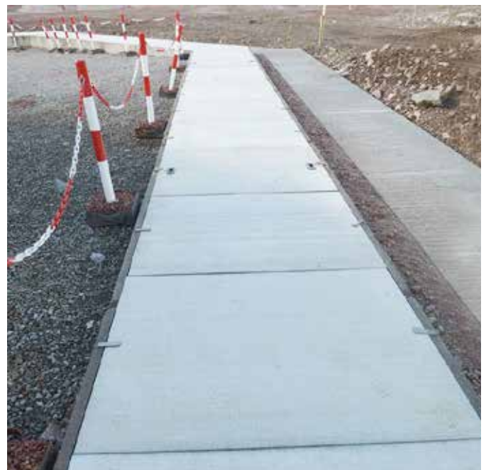
Concrete covers unable to withstand pedestrian traffic
