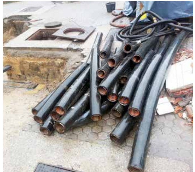
The previously installed steel piping had less flexibility than KPS piping
