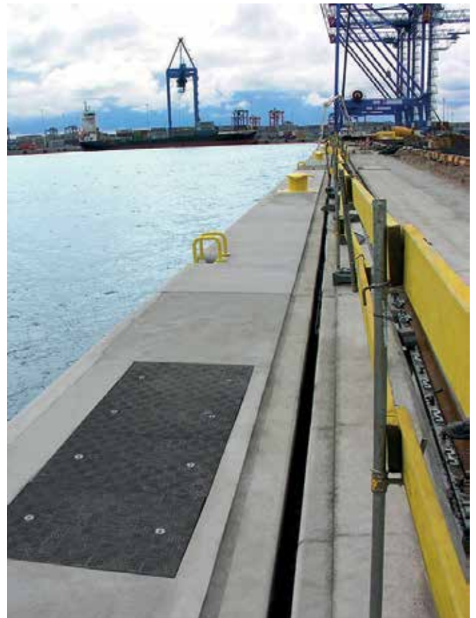
Fibrelite's trench covers covering access pit
