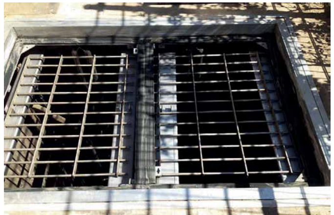
Removable beams hold safety grid
