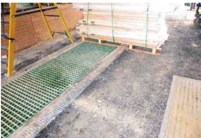
Previously installed GRP grating was originally supplied together with the precast concrete troughs
