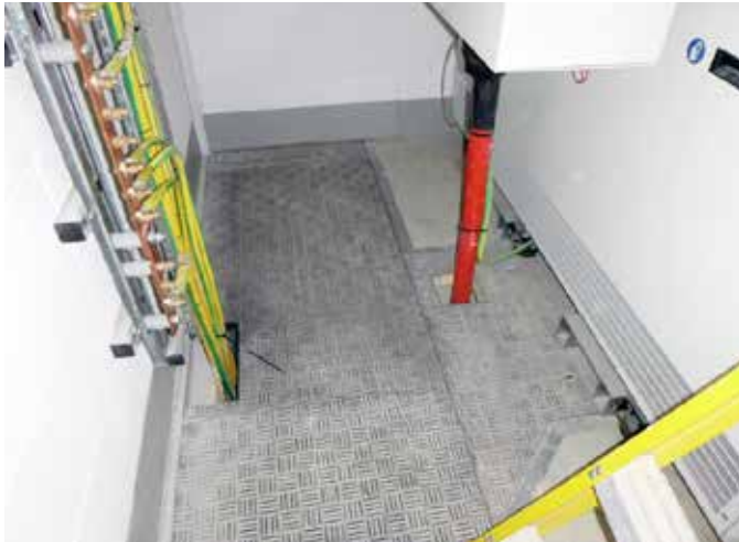
Bespoke Fibrelite GRP composite access covers installed at pharmaceutical facility in County Durham
