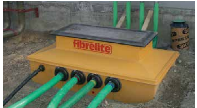
Fibrelite's vapour recovery transition sumps being vacuum tested to ensure a watertight installation
