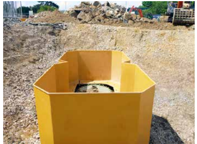
The new double chamber fit to the previously installed split container tanks
