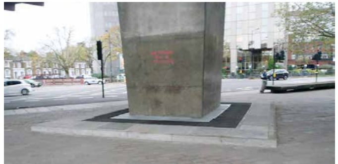
Roller bearings at the bases of supporting piers were replaced due to wear and increased load on the bridge
