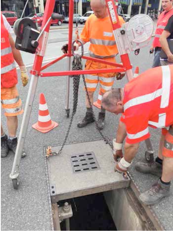
Previously installed heavy (15cm thick) concrete/steel infill covers
