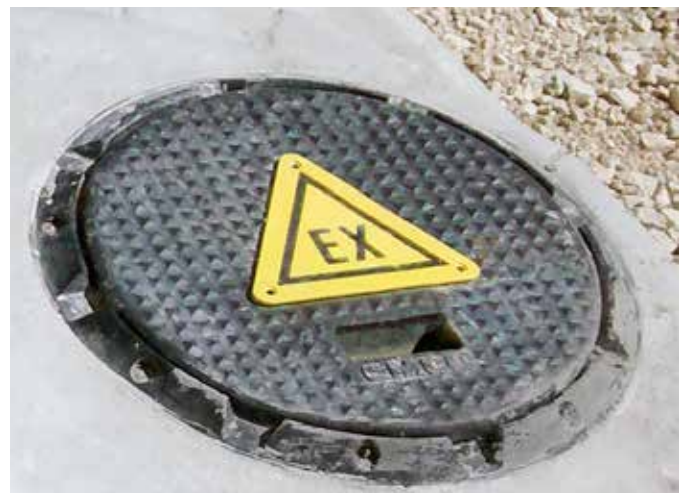
Previously used cast iron spill chamber
