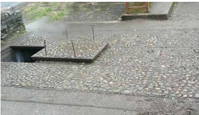
Cobbled covers requiring lifting equipment
