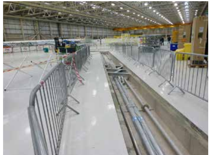
Essential service pipework required for the production process
