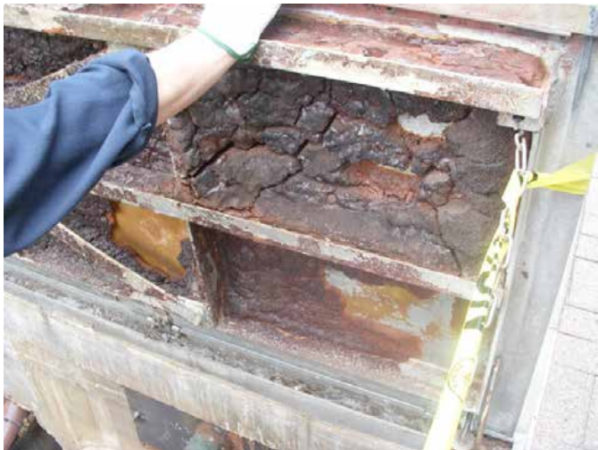
Degraded thermal insulation beneath the old aluminum vault covers
