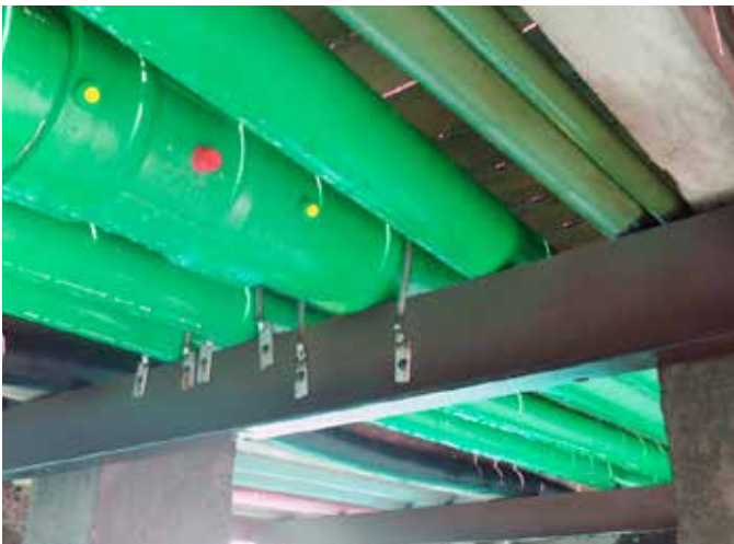
Fuelling lines run below jetty from ship to storage point
