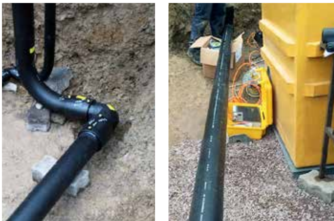
Petro Systems Management's first site using KPS piping
