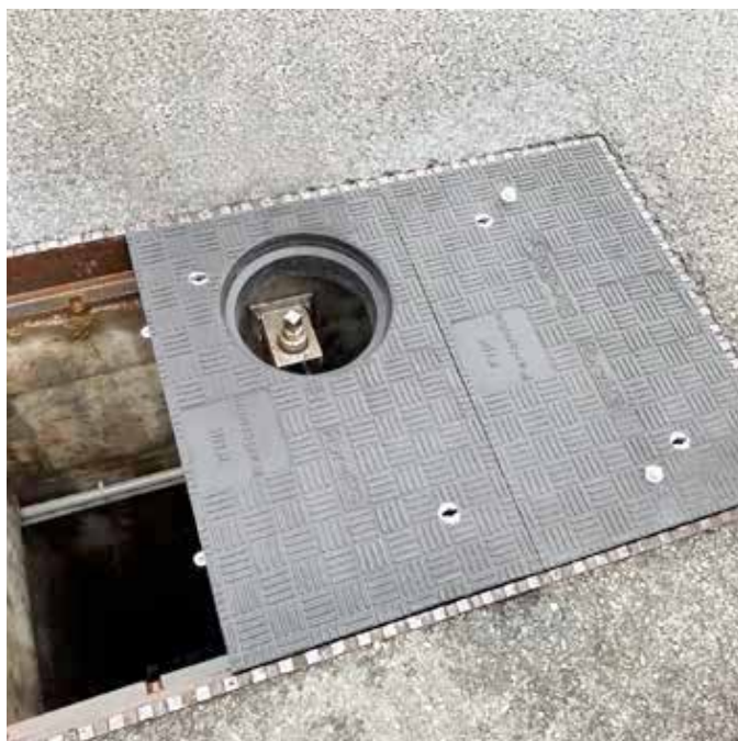
Custom Fibrelite covers retrofit into existing frames, including an inspection port exactly over the slider
