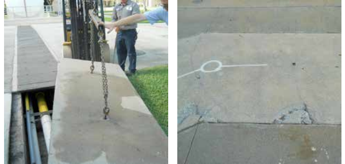
Traditional concrete panels are unsafe and labor intensive to remove and often break apart over time
