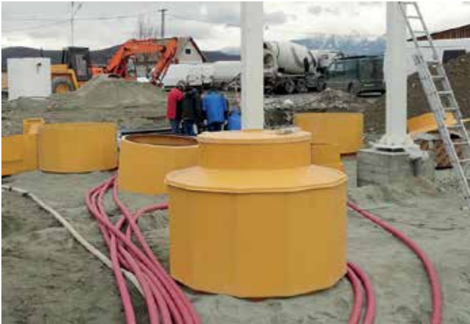
Gazprom have specified Fibrelite's fully conductive 1.6m dia chambers (S16) to facilitate easy maintenance post installation
