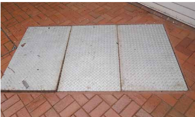
Previously installed odour-emitting galvanised covers
