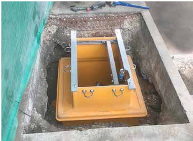
BP required retrofit chamber systems
