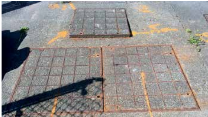
Covers were showing signs of severe corrosion
