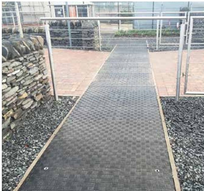
Newly fitted pedestrian traffic trench with anti-slip resistance as standard
