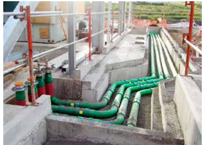
OPW provided a compact solution combining KPS piping and Fibrelite sumps
