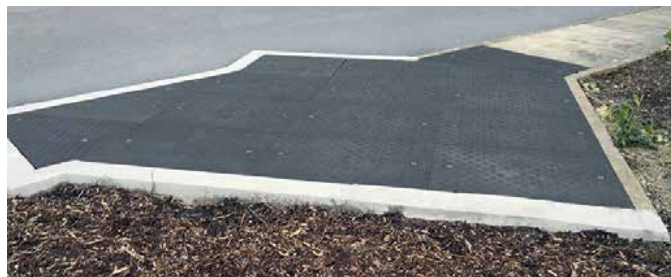
Bespoke "cassette" of Fibrelite covers and supporting steelwork installed to tight construction deadline
