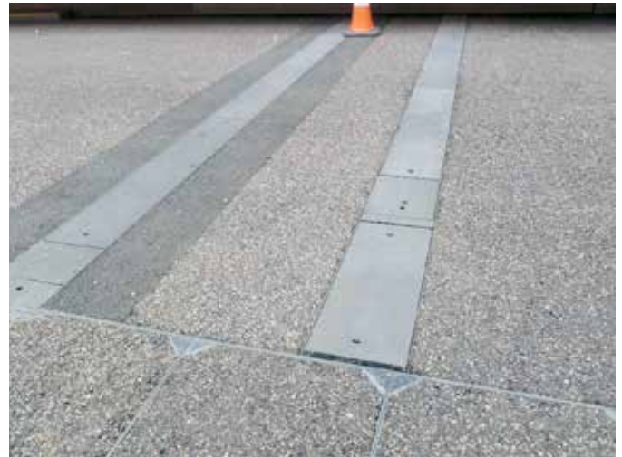
Previously installed covers were unable to withstand heavy loads causing them to crack and deform
