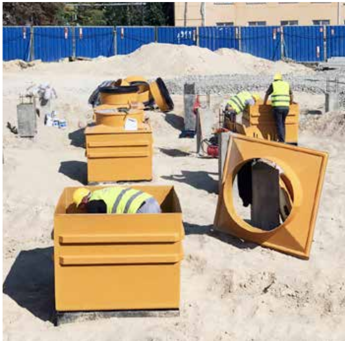
Technical support and installation training was required on site to complete the project within its tight timescale
