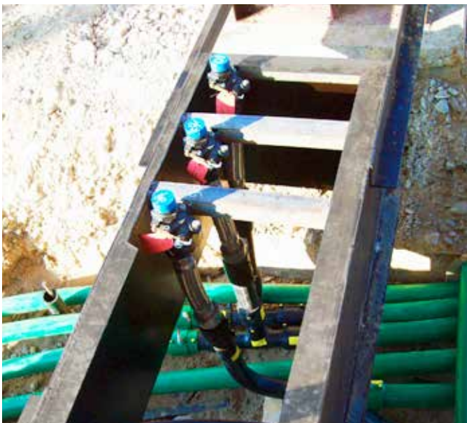
Sinooil required a solution that allowed emergency valves to be installed under dispensers
