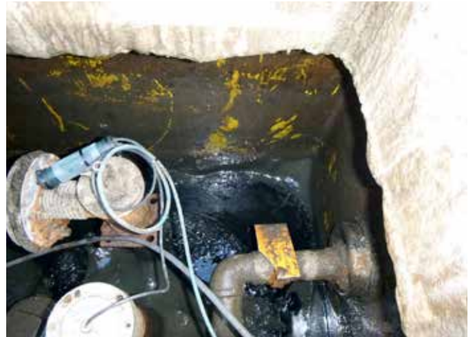
Previously installed chambers had corroded, allowing water ingress
