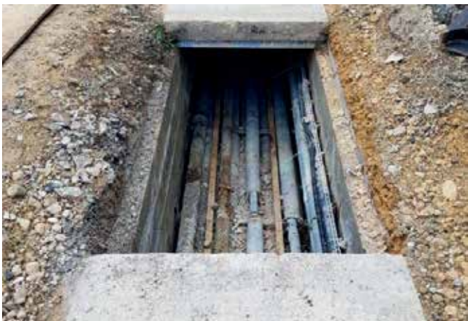
Fractured covers had allowed dust and debris to enter the trench
