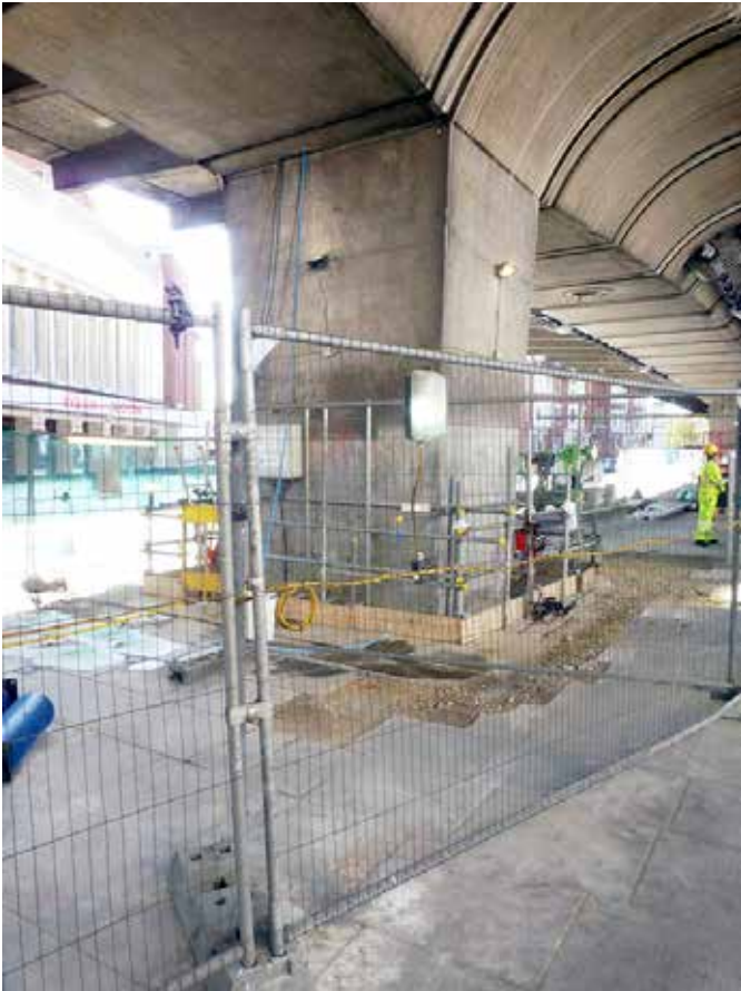
Roller bearings at bases of supporting piers before being replaced
