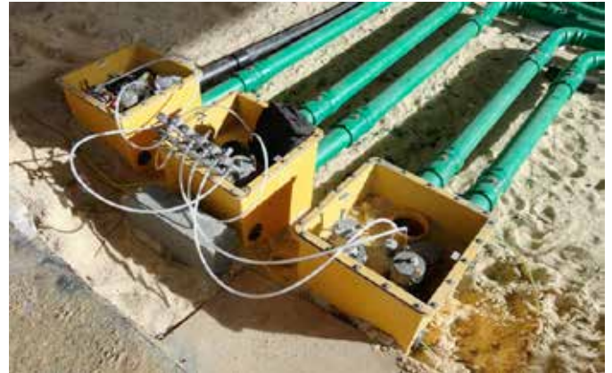
Secondarily contained Fibrelite remote fill sumps
