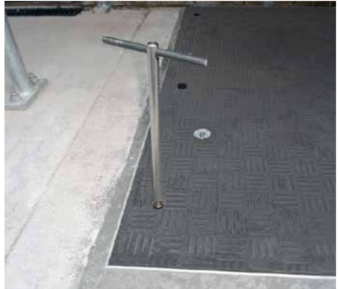
Secured/restrained covers, preventing unauthorised access
