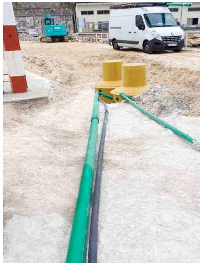
Conductive pipes avoid any static electricity build up from fuel flow
