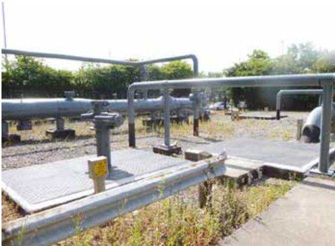
Cadent Gas Valve Pits, North West England
