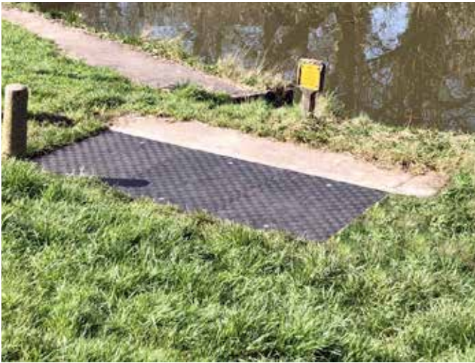
Fibrelite covers continue to be installed at Cadent Gas facilities across the UK
