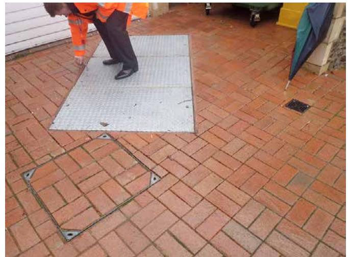
Unsafe lifting of the old covers - health and safety hazard
