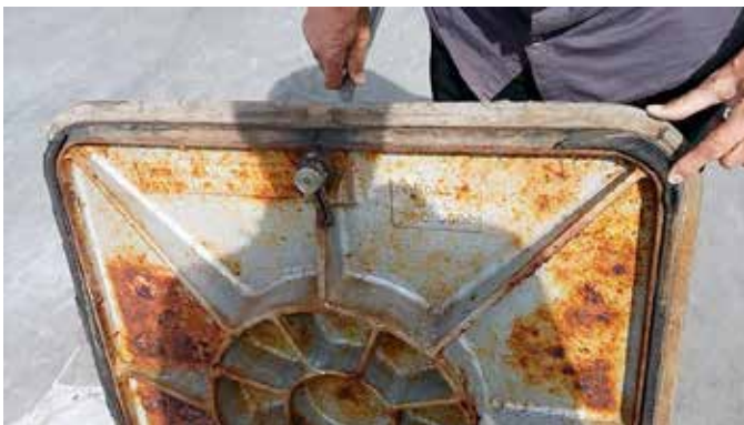
Failed seal due to rust allowing water ingress into chamber
