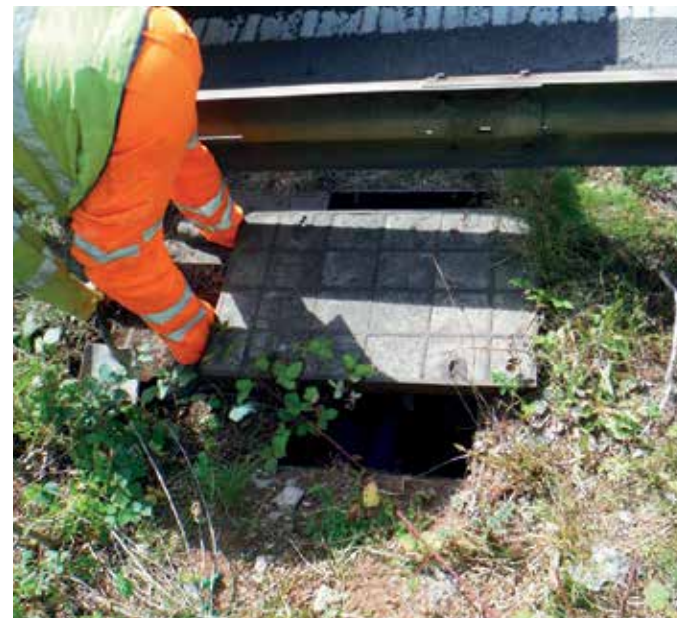
Damaged cast iron and concrete cover
