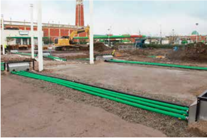
10m lengths of custom 75/63mm KPS straight pipe allowed fast installation without the need for a welding socket in middle
