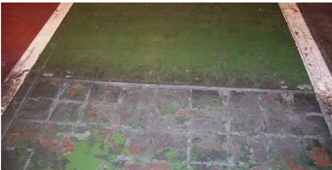
Once removed the concrete covers would never sit back in the frame correctly
