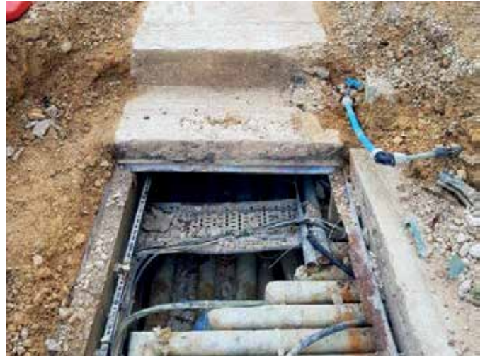
Concrete covers posed a risk of injury to maintenance workers due to their weight
