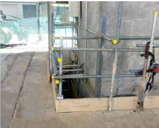
Spherical sliding bearings located in underground pits, allowing for minor movement of the pier
