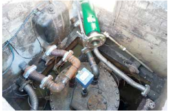
A hole was cut in the corner of each sump to allow the KPS termination fittings to enter
