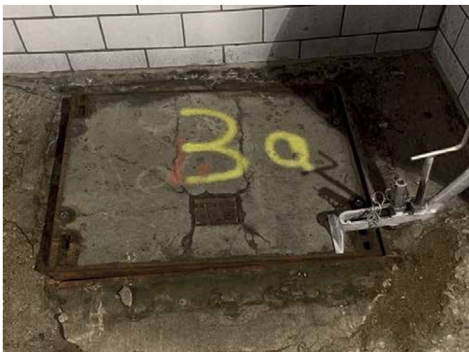
Old unsafe concrete covers
