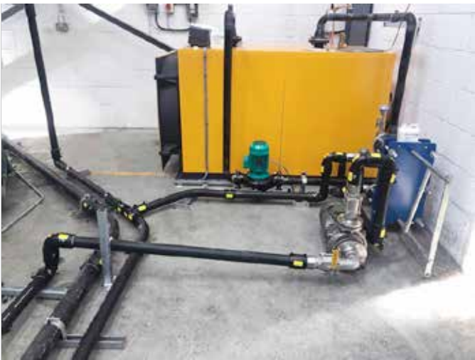
A piping system with a large range of fittings was required
