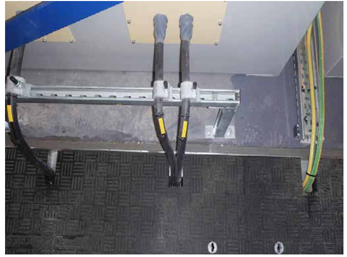
Custom made covers fit the trench and cabling entry points perfectly
