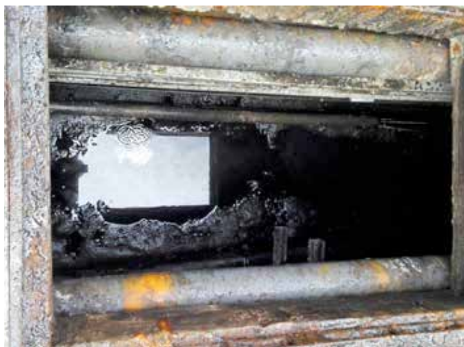
Due to the corrosion, the pipes had begun to break down
