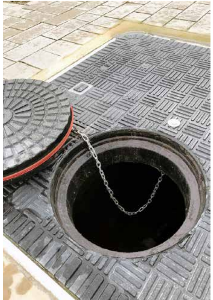
The Fibrelite cover that was installed can be easily removed by one person
