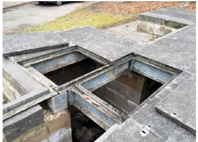
The previously installed obtrusive framework made access difficult and led to health and safety risks
