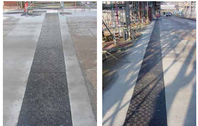
The senior designer on site commented that everyone was very pleased with the finished result
