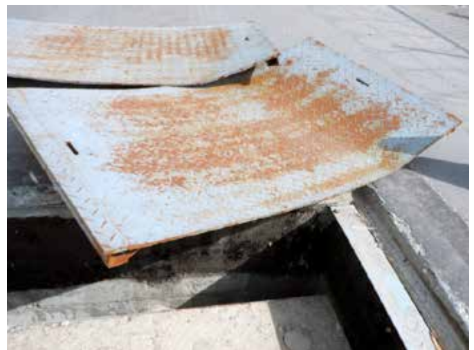
Covers had begun to rust and degrade due to the harsh field conditions
