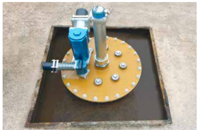
OPW's Fibrelite team came up with a solution to chemically bond the GRP square chambers onto the old tank upstands
