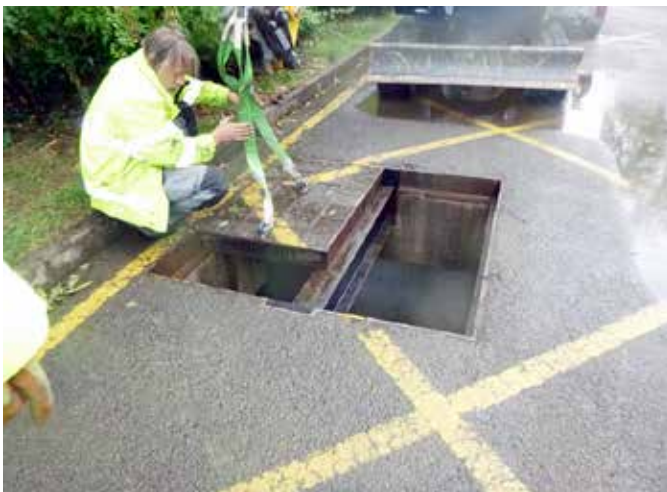
Due to the weight and difficulty in removing the covers critical time is lost in emergency situations
