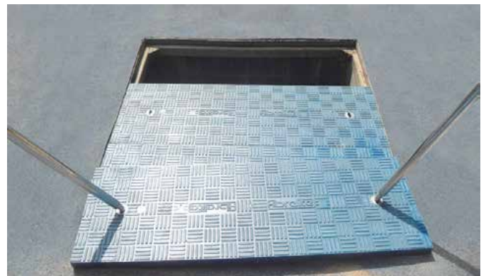
The recently installed Fibrelite coloured trench covers
