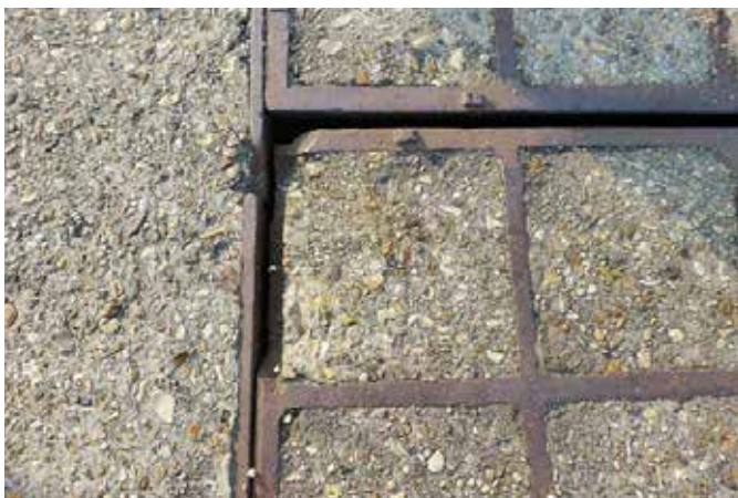
Corroding previously installed covers
