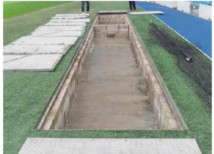
A camera pit to be covered by Fibrelite composite trench covers
