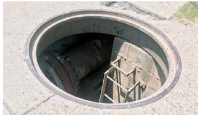
The previously installed cover had made access to the vault difficult
