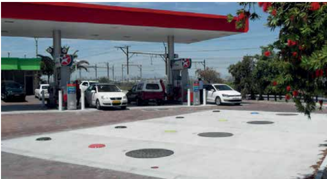
Recently upgraded site with Fibrelite's 900mm covers (FL90's)
