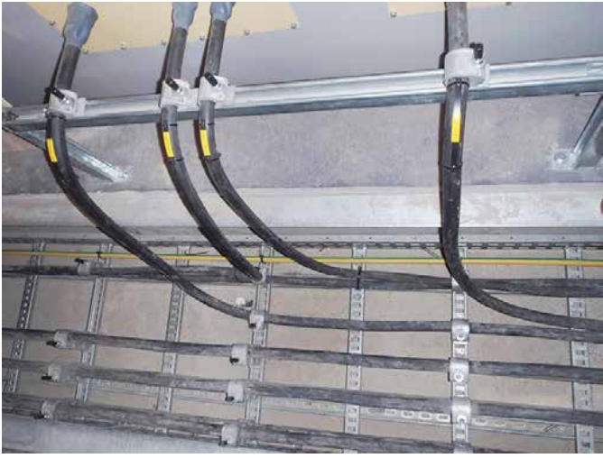
Expansive trench requiring coverage
