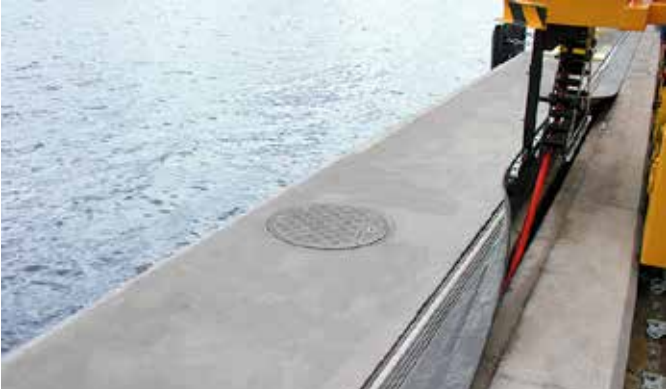
F900 load rated sealed cover over fresh water valve pit
