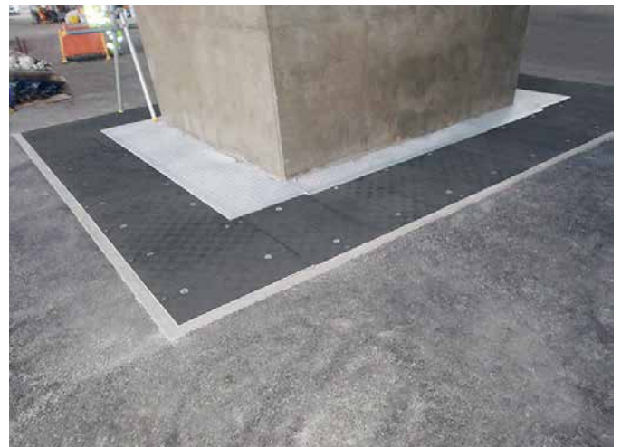
Replacement bearings located in the underground pits, covered by continuous set of access covers, allowing for the minor movement of the pier
