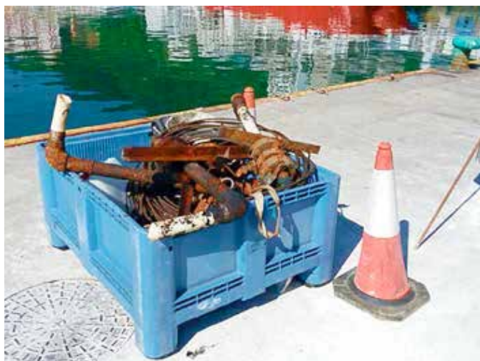
Previously installed metal piping had corroded due to the salinity of the water
