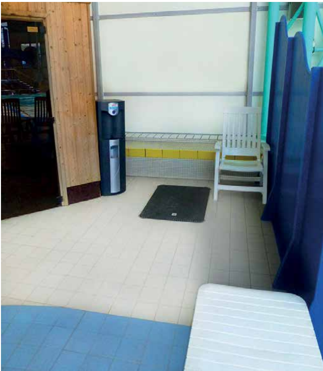
Leisure centres are highly corrosive environments with moisture and chlorine, making composites an obvious choice
