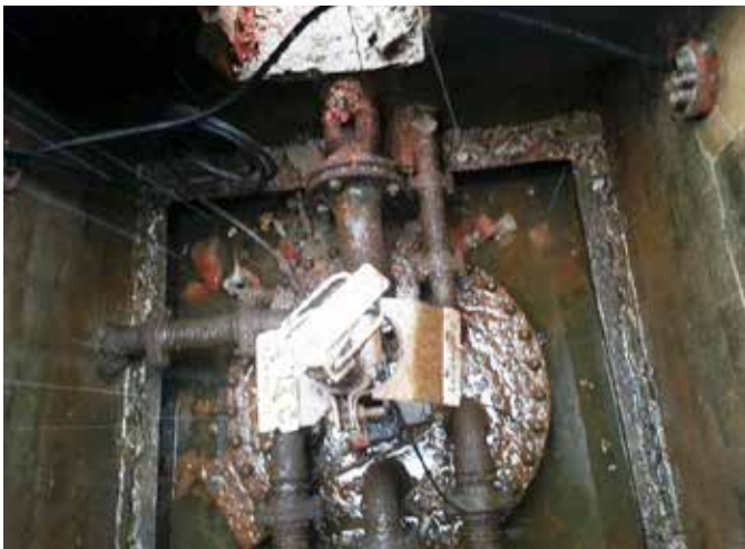
Previously installed steel piping had become damaged over time and started to rust
