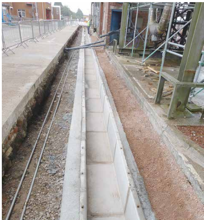
From an initial website search for lightweight composite panels to the installation of 190 new Fibrelite covers
