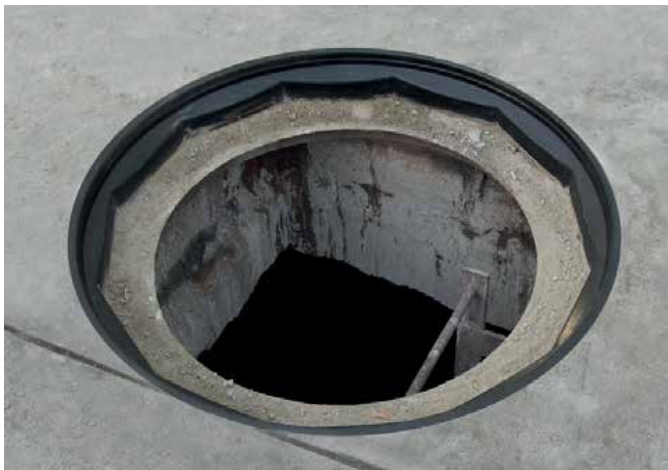
Fibrelite composite frame installed in sidewalk
