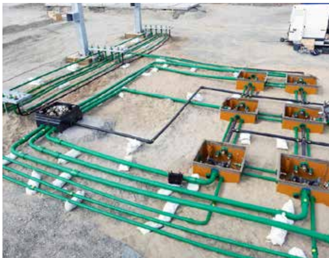
KPS piping had to be installed within 5 working days to meet the strict project deadline
