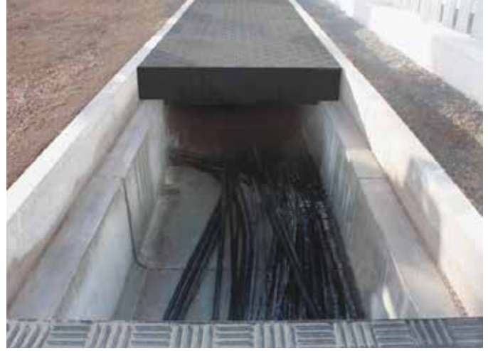
Slit trench with stepped covers over electrical cabling
