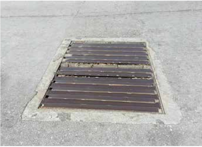
Modular metal covers time consuming and hazardous to remove due to weight, multiple sections and corroded edges
