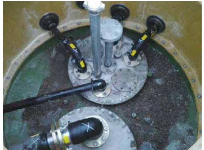
Fibrelite's latest tank sump design installed on CGH Nordic storage tanks
