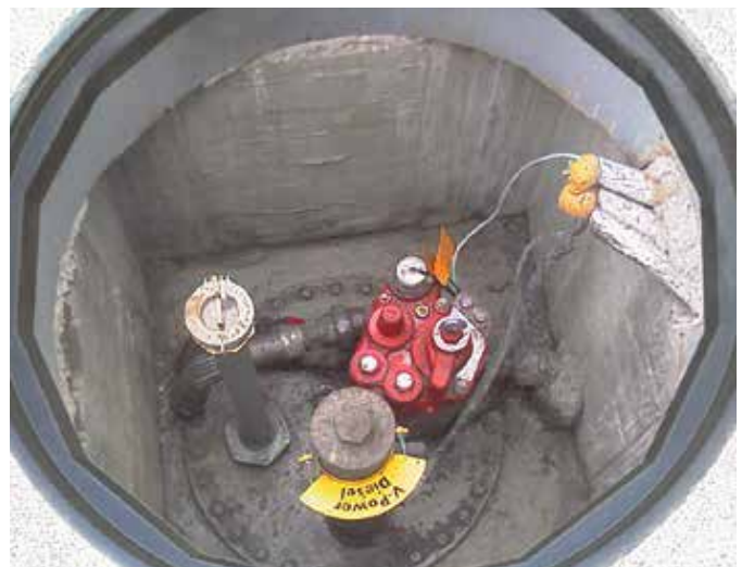
Fibrelite's covers prevented surface water ingress into chambers above the fuel tanks
