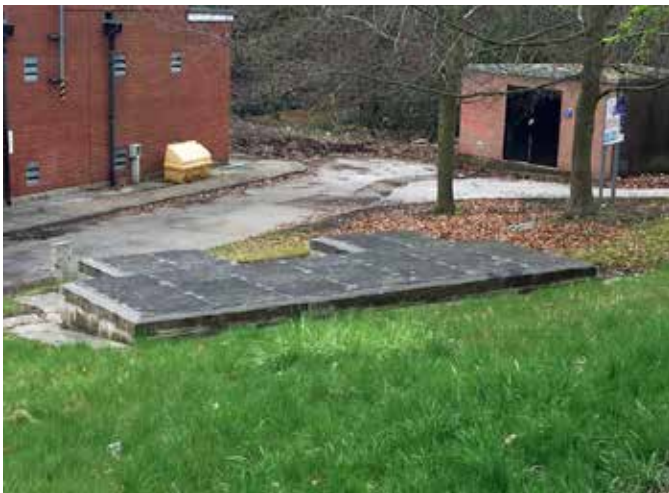
RJ Utilities required trench covers that would improve the efficiency and safety of the site
