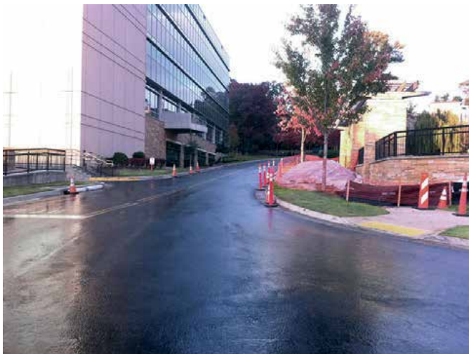
Pre-install location for the Fibrelite covers
