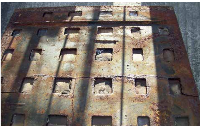
The previously installed old corroding and crumbling concrete covers
