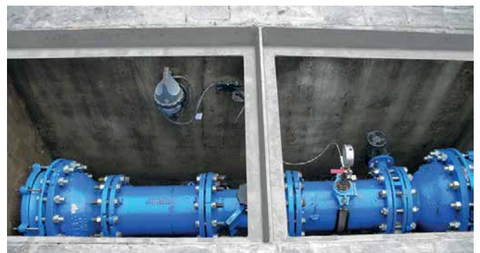
Fibrelite trench covers fitted into existing frames, preventing expensive breakouts and time for concrete to set (Image credit: Aguas de Cádiz)
