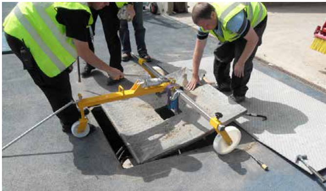
Manual handling: the previously installed damaged cover required a hydraulic lifter to remove the cover
