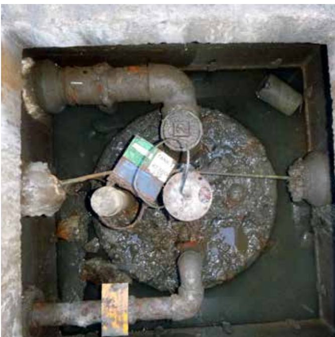
At this site, the old tank upstands were too small for the traditional bolt down chambers tank sumps / chambers
