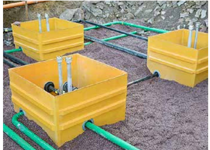
When the first site was under construction, the OPW team were on hand to offer onsite installation and guidance
