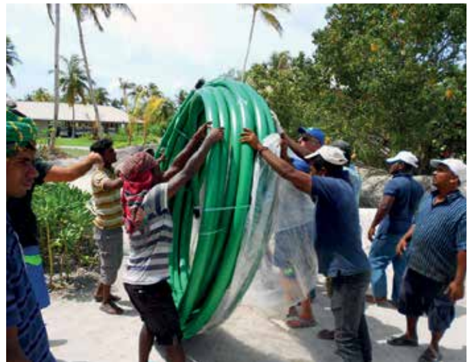
Unwrapping the KPS 75/63SCEC double wall fuel coil for the new fuel line
