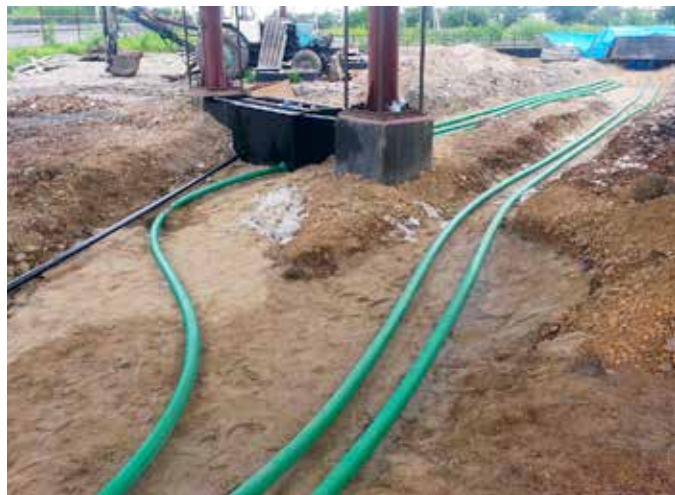
The customer now has a long-lasting KPS solution that will continue to perform year after year
