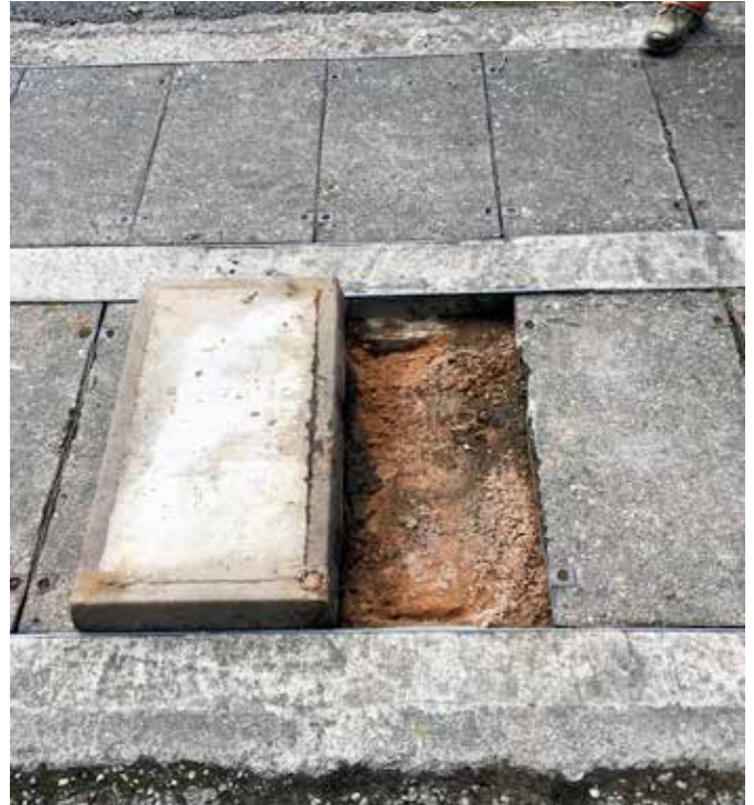
The previously installed covering arrangement was deteriorating
