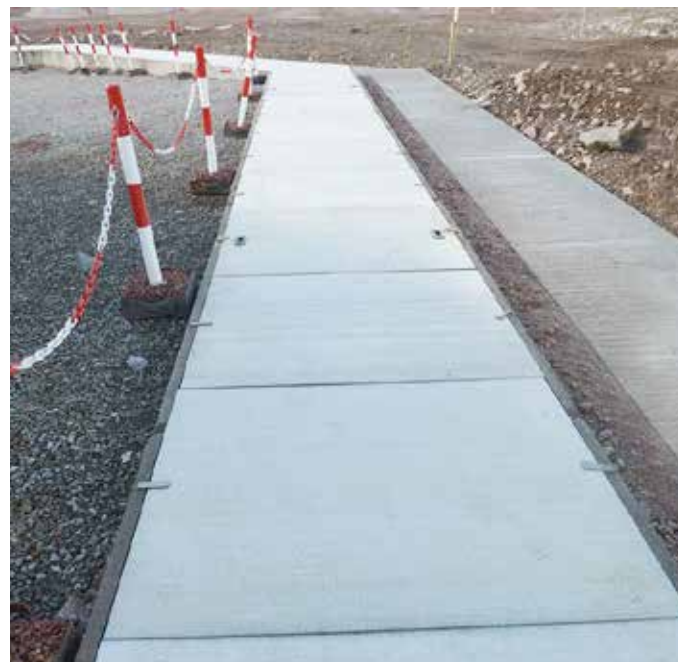
Concrete covers unable to withstand pedestrian traffic
