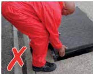
Dangerous lifting technique without Fibrelite lifting aid
