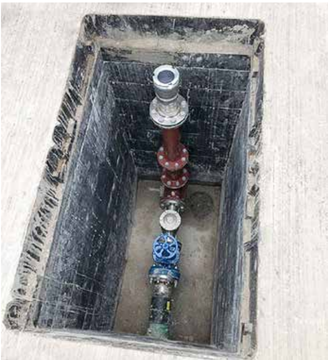
Complete below ground remote fill point
