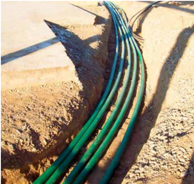
KPS provided long-term plastic piping system for pressure lines in Kazakhstan
