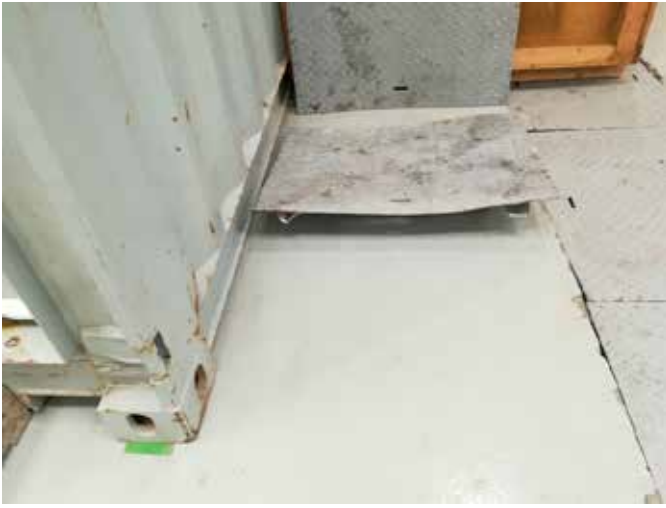
The steel covers had buckled under the load
