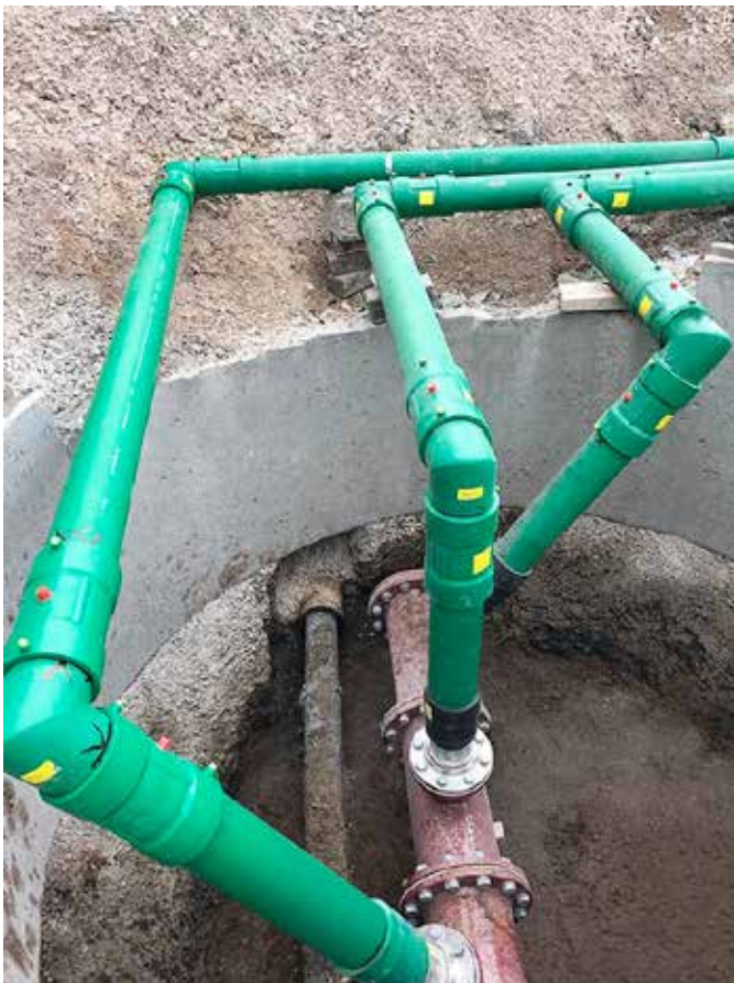
Compact moulded elbows make the join from new KPS piping to the previously installed fuel piping
