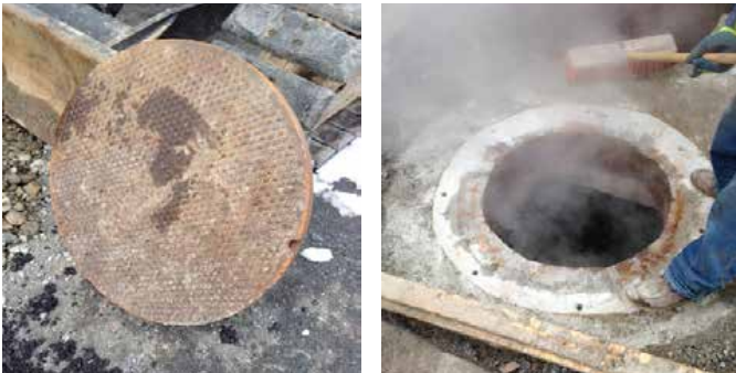
Large cast iron covers are both very heavy and extremely hot when exposed to steam within the manhole
