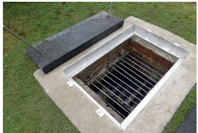
Safe and easy manual removal: Fibrelite FM45 covers are removed by hand from the CSOS (Combined Sewage Overflow System) chamber
