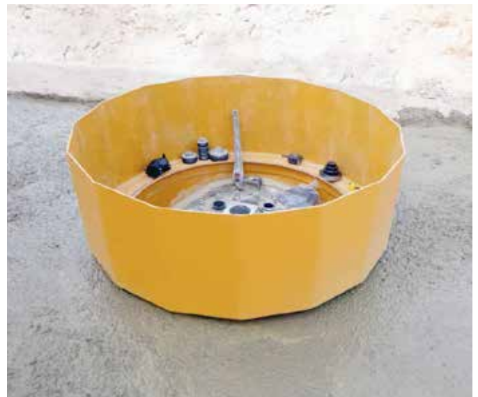
An epoxy putty compound was used to bond the collar directly to the tank
