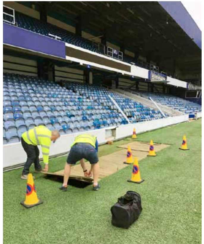
The existing covers had become a major health and safety hazard, with covers considered unsafe for pedestrians
