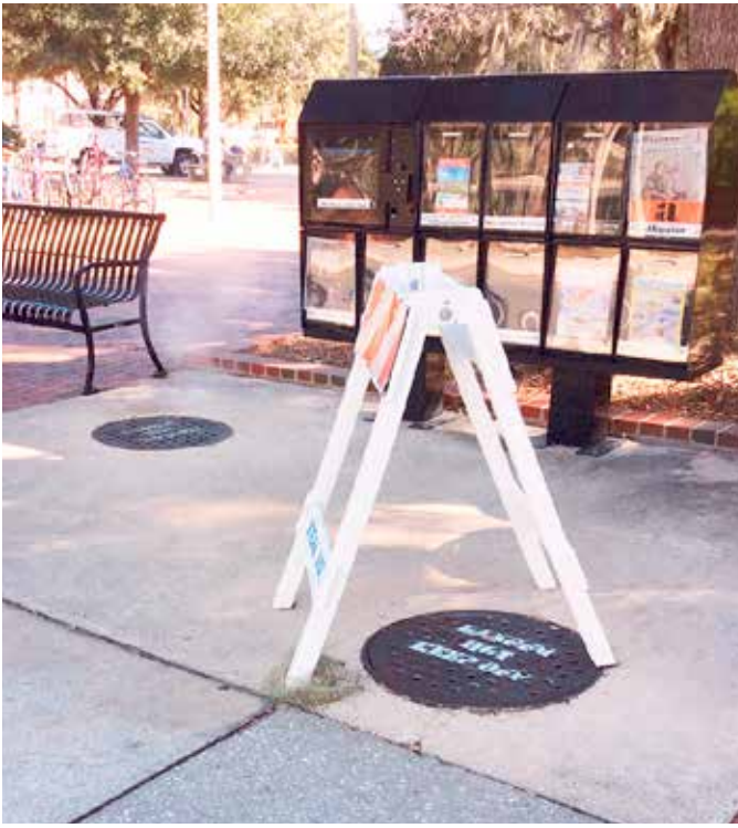
Original cast iron covers at the University were blocked because of their high temperatures due to steam.
