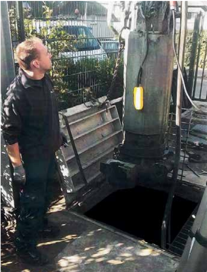
Heavy metal covers requiring 2 men and a crowbar to remove, emanating odours
