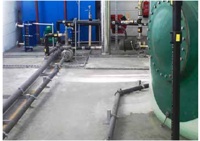
KPS piping is made of high-density polyethylene, and includes liners to prevent permeation of fuel
