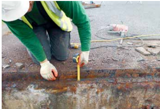
Previously installed heavily corroded access covers
