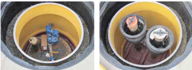
Fibrelite turbine and fill sumps
