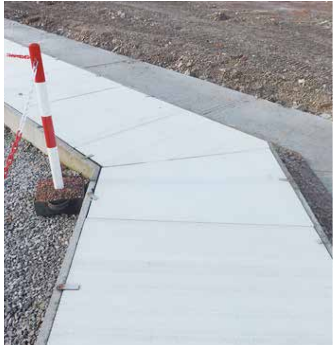
Previously installed low quality concrete covers
