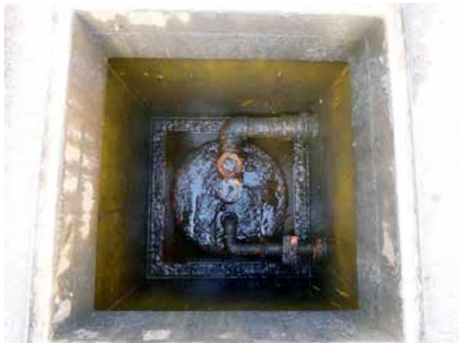
Previously installed chambers allowed water ingress
