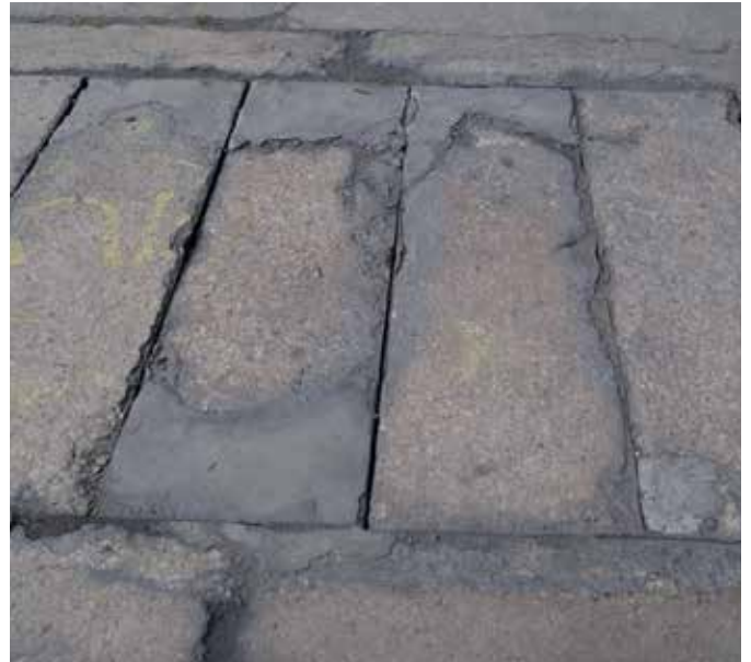
Damaged and difficult to remove: heavy concrete slabs
