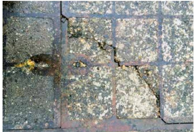
Deep cracks had formed in the corroded previously installed covers
