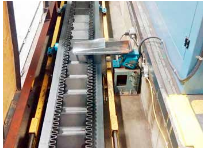
Underfloor conveyor in trench takes products from presses to packaging
