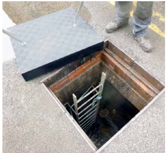
The covers provided access to underground water valves
