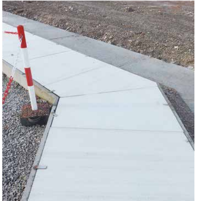
Previously installed low quality concrete covers
