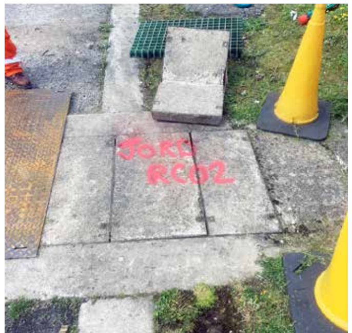
Covers were extremely heavy to lift
