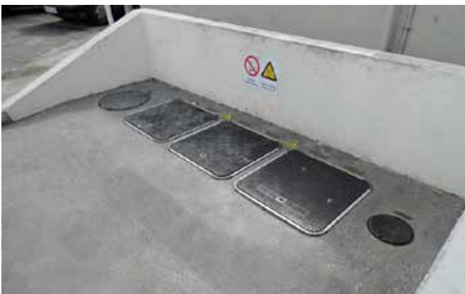
Recently upgraded site with Fibrelite's 600mm sq. 25 tonne load rated covers (FL60)
