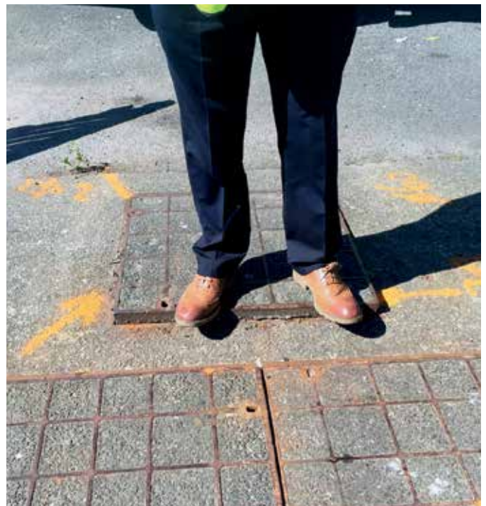
Previously installed heavy concrete recess covers were showing signs of severe corrosion
