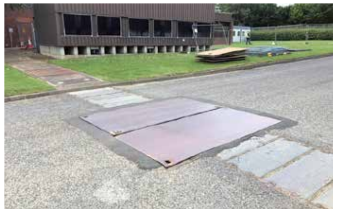
Sheets of metal had been installed as a temporary patch over failing concrete covers
