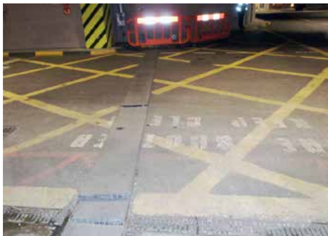
Previously installed covers were poorly fitting in their frames due to the covers being distorted.
