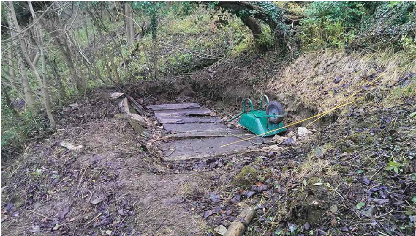
Old heavy slate covers posed a lifting hazard when access was required
