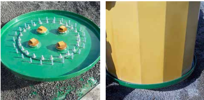
Fibrelite's 42" E85 compatible tank sumps being installed on double wall steel tanks
