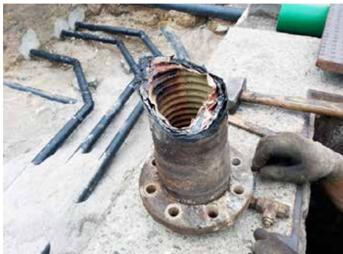
Previously installed corrugated steel and copper piping was damaged due to corrosion
