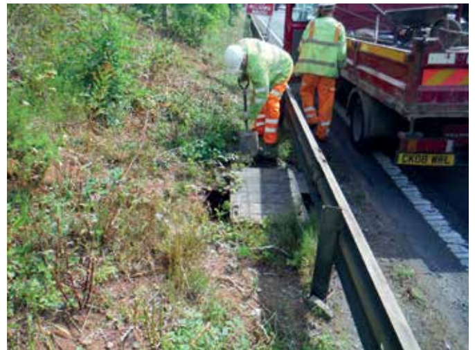
Heavy covers present a hazard for operators
