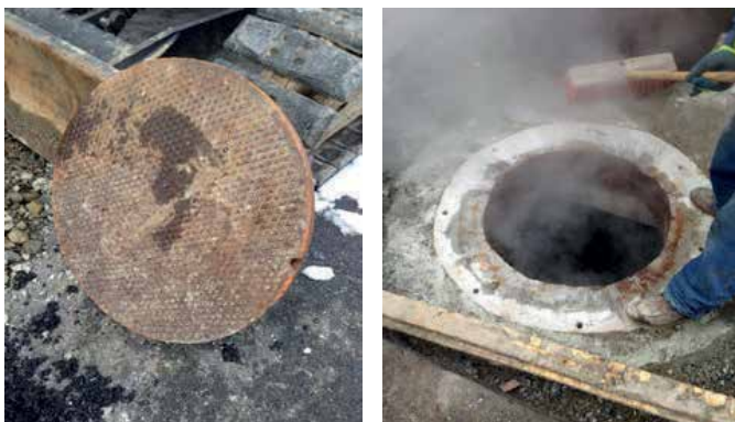
Previously installed large cast iron covers were very heavy and extremely hot when exposed to steam within the manhole
