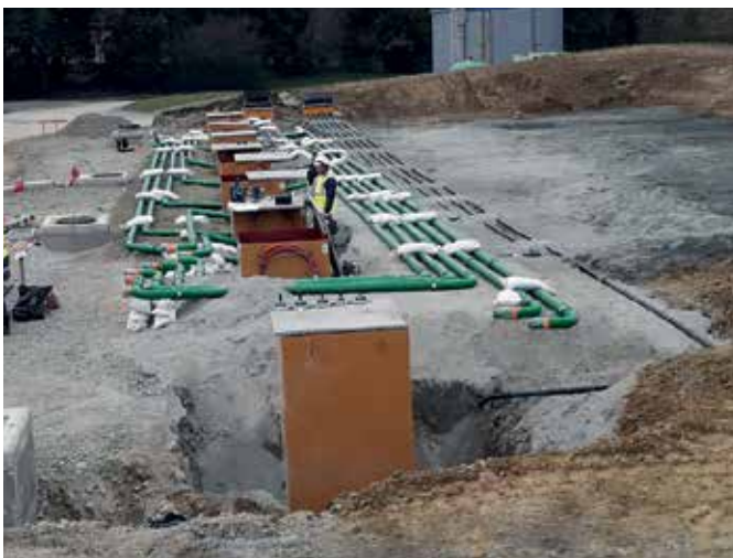
OPW provided a tailor-made KPS piping solution
