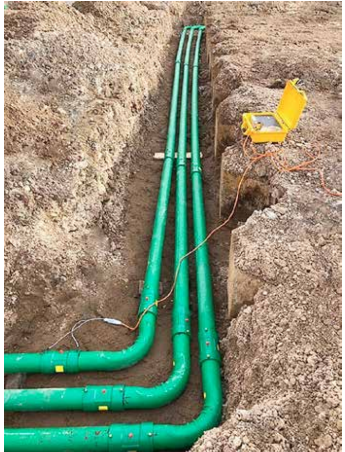
KPS double wall diesel piping
