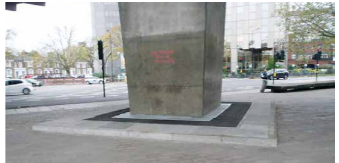
Roller bearings at the bases of supporting piers were replaced due to wear and increased load on the bridge
