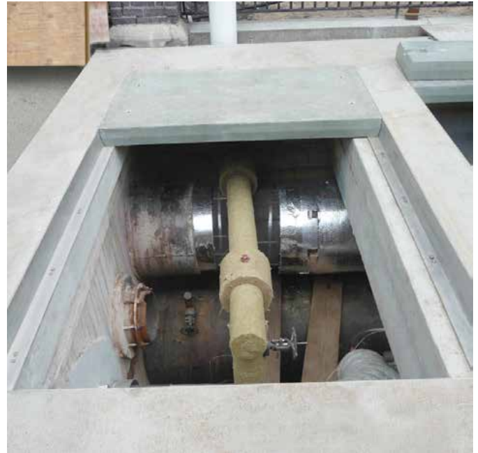
Six Fibrelite FM45 4' 6" (1.6m) wide anti-slip GRP composite trench panels being installed in the sidewalk
