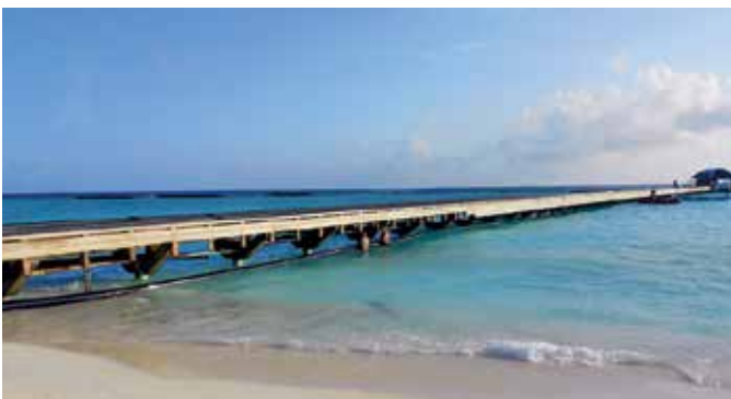
Fuel delivery jetty: piping has constant exposure to saltwater
