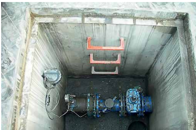
Automatic monitoring system located beneath metal cover which blocked signal (Image credit: Aguas de Cádiz)
