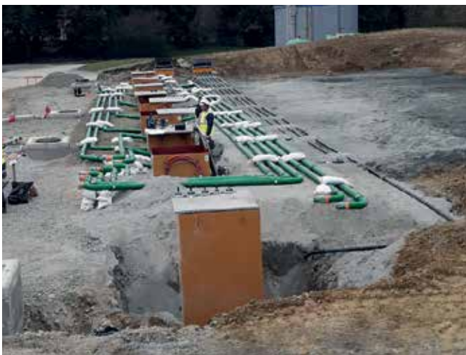
OPW provided a tailor-made KPS piping solution
