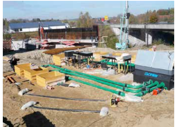
OPW provided a complete sealed system for ENI Germany
