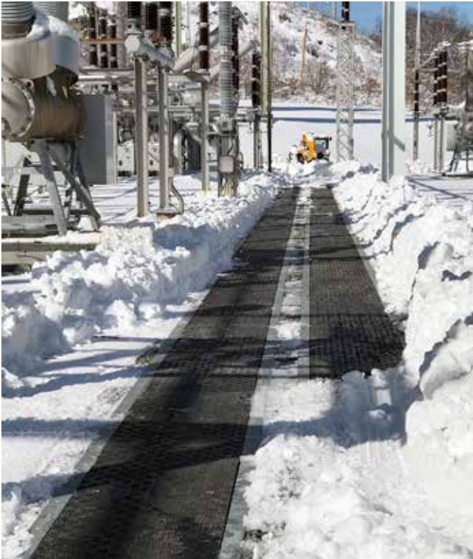
Custom HS20 Fibrelite covers in Trenwa's precast concrete trenches
