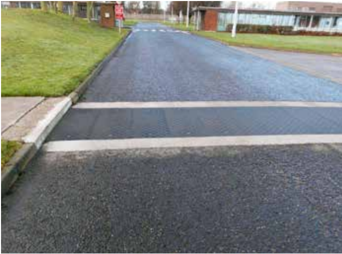
Fibrelite GRP access covers installed at pharmaceutical facility in Northumberland, UK
