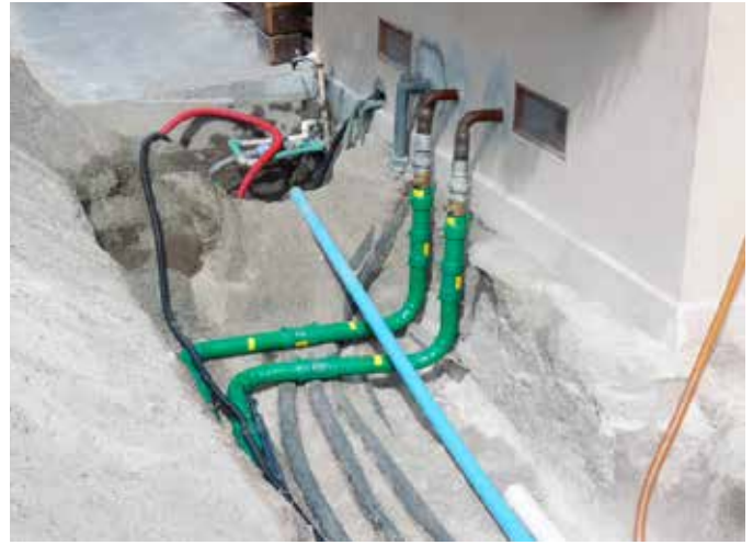
Refuelling lines running from storage point to jetty
