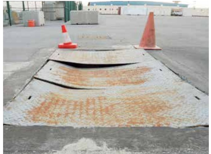
As a result of deformation and corrosion of the covers, dust and debris were entering the trench
