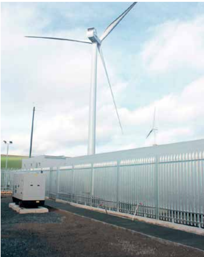
Fibrelite D400 trench covers on wind farm substation
