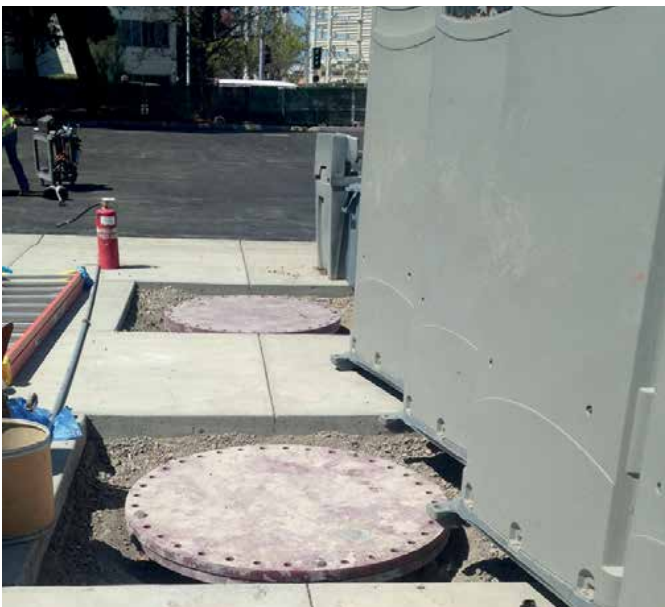
Fire manway lids (tank buried underneath)
