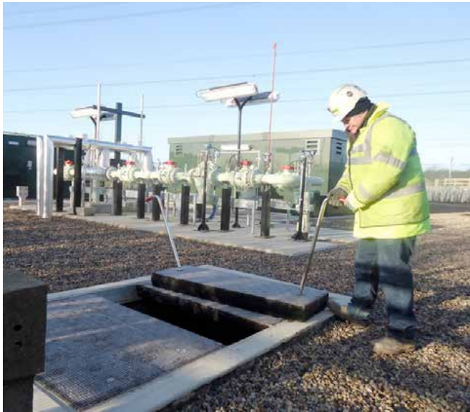
Easy and safe access to underground systems
