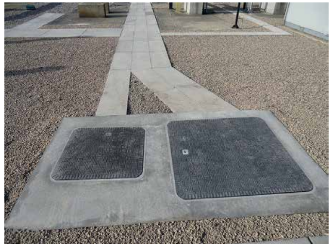
Fibrelite's watertight sealed manhole covers installed
