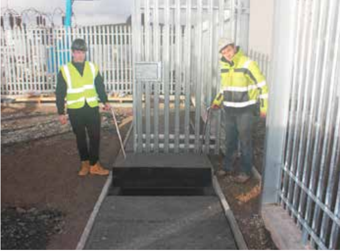
Covers safely manually removed with Fibrelite's ergonomically designed lifting handles
