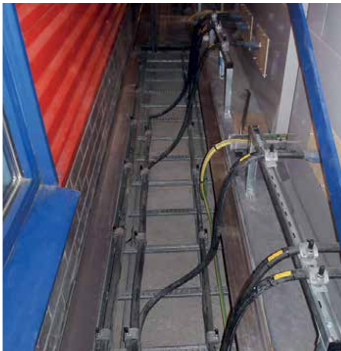
High and low voltage cables leaving trench to switchboard at regular intervals
