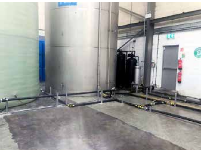
This project had a tight build schedule, so installation time was key
