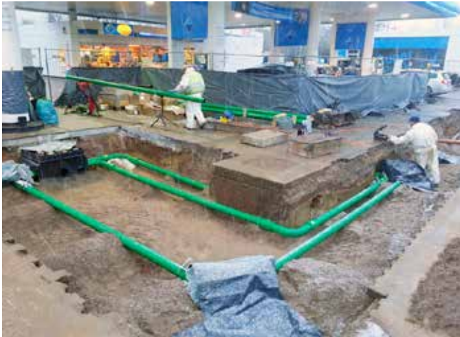
KPS' quick and easy installation resulted in no interruption of fuel sales
