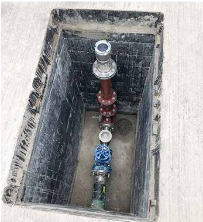
Complete below ground remote fill point
