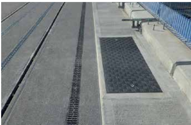
Bespoke trench covers for trackside gear
