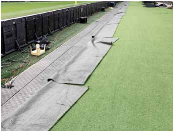
Bespoke Fibrelite GRP trench covers installed over electrical cabling trenches
