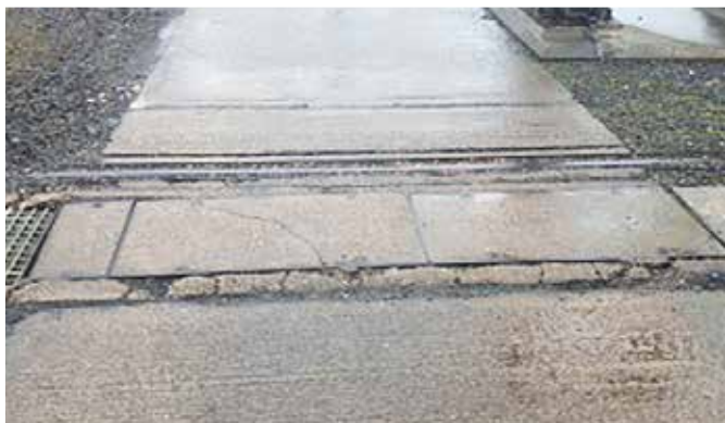
The previously installed cast iron frame showing signs of damage and corrosion
