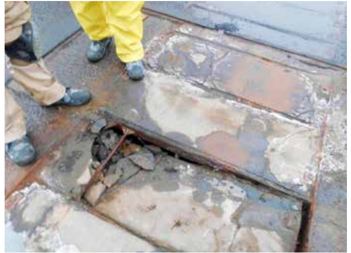
Heavily corroded previously installed covers
