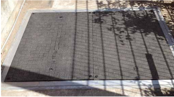
Sealed odour-tight covers installed
