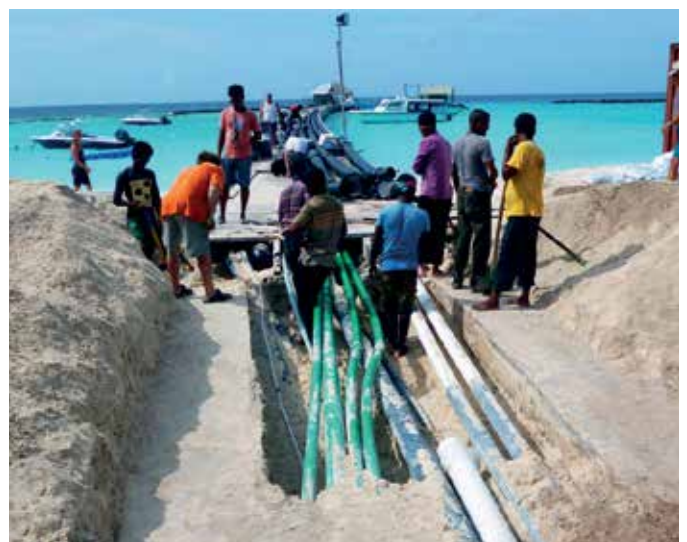
Installer friendly KPS piping allowed for quick easy installation
