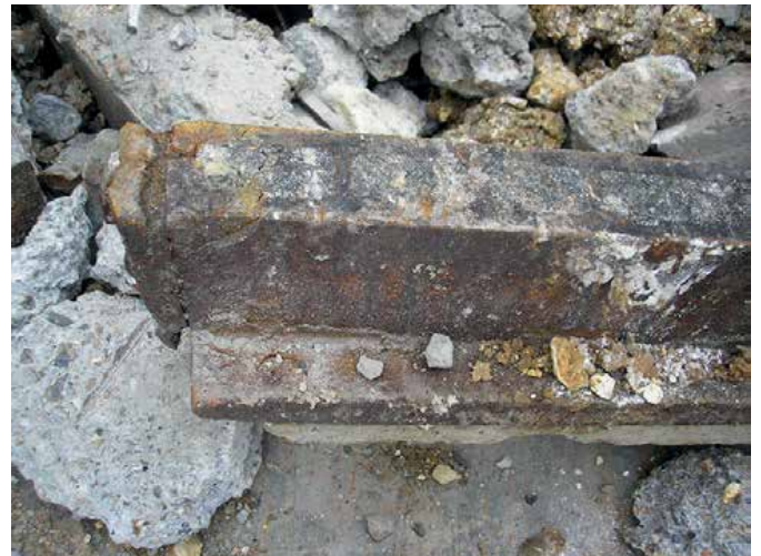
The previously installed cast iron frame showing extensive damage and corrosion
