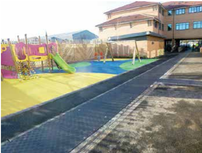
James House in York required a strong, lightweight long-term solution to cover their PCC troughs
