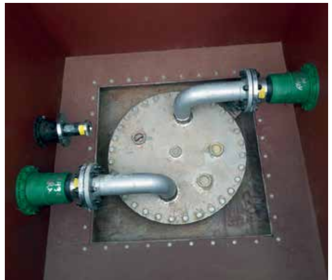
Fibrelite vent transition sump provided easy access to KPS single wall suction system and double wall suction system (pictured)
