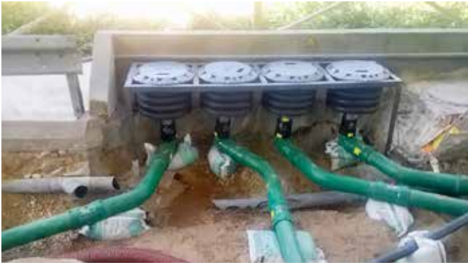
Cast iron chambers often have to be fixed in a frame and piping supported (pictured: different site to show possible frame configuration)
