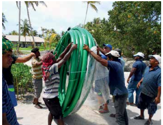
Unwrapping the KPS 75/63SCEC double wall fuel coil for the new fuel line
