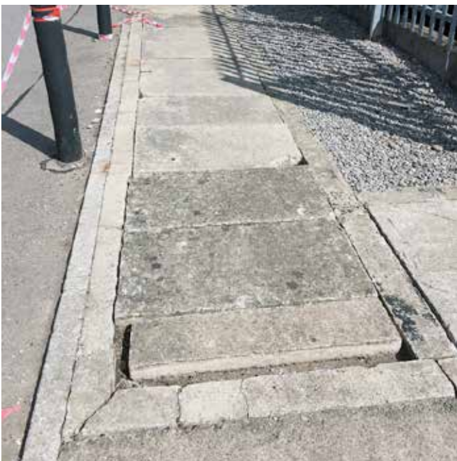
Previously installed failing concrete trench access covers
