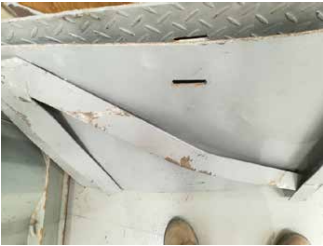
Previously installed covers had also begun to corrode
