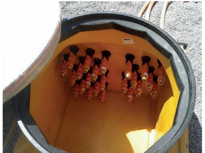
Cable drawpit with 32mm conduit piping
