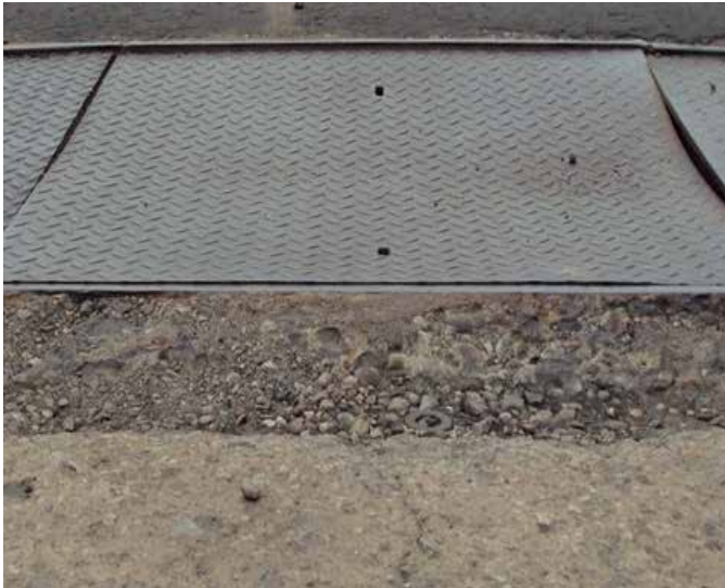
Corroded and deformed cheap steel covers
