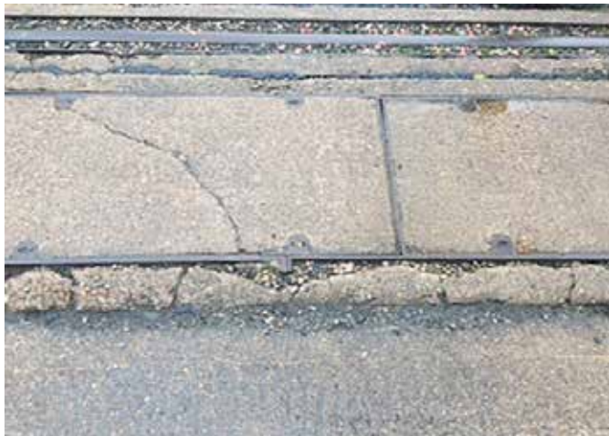
Previously installed corroded and damaged cast iron and concrete covers
