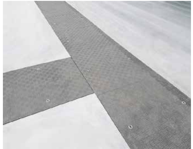
Fibrelite and Corrimex installed a T junction as a part of the project
