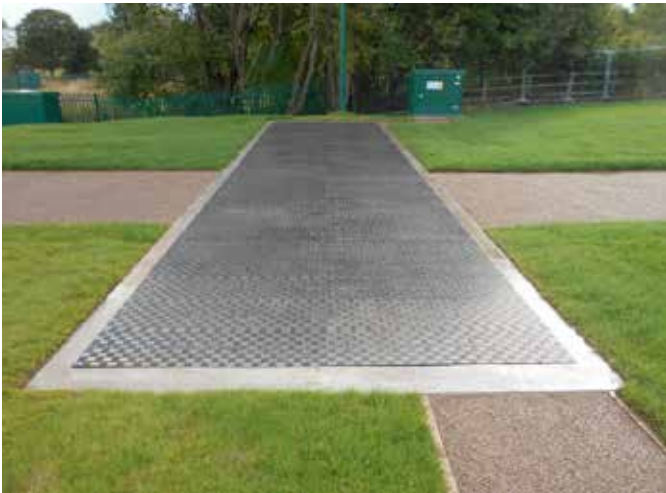
The Fibrelite B125 (12.5 tonne) load rated medium duty trench access covers installed
