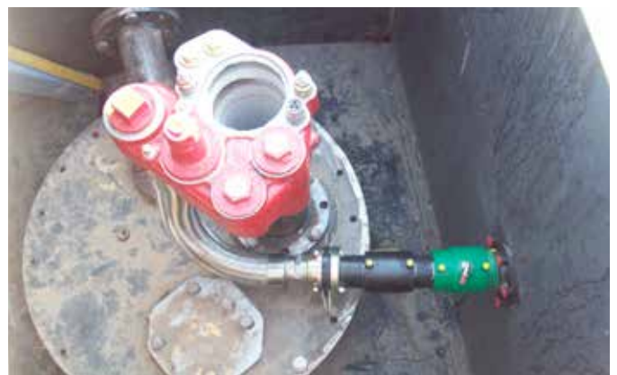
The KPS compact solution allowed for emergency valves to be installed under dispensers
