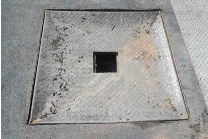
Out with the old: the damaged reinforced steel cover to be replaced by Fibrelite's trench covers
