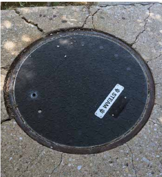
The previously installed covers locking mechanism had failed due to the heat
