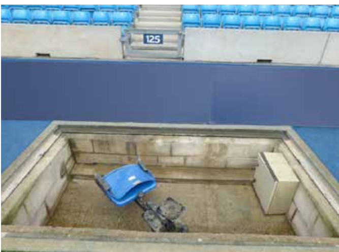
An existing camera pit to be covered by Fibrelite's composite trench covers
