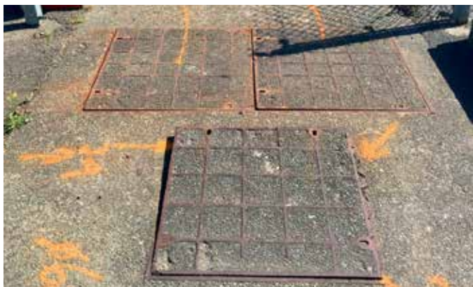
Previously installed heavy concrete recess covers
