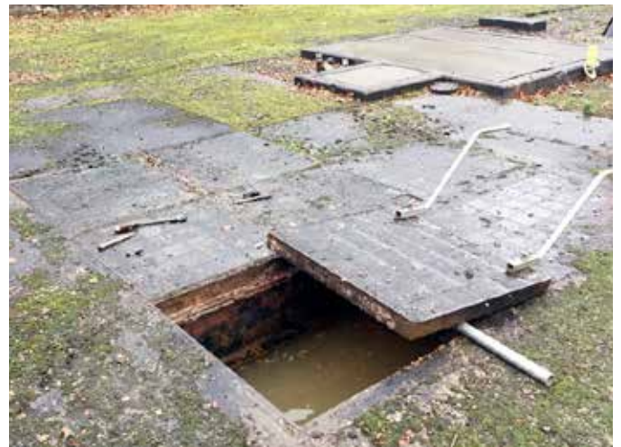
Previously installed covers were extremely difficult to remove and replace safely
