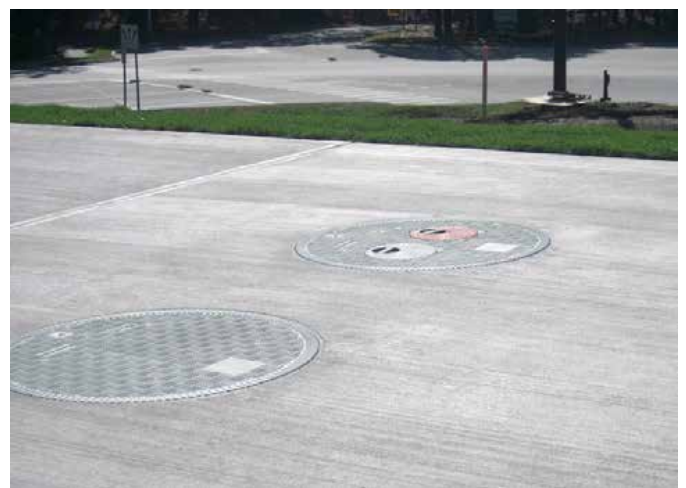
Tank pad showing FL100-MP Fibrelite multiport cover and FL100 cover
